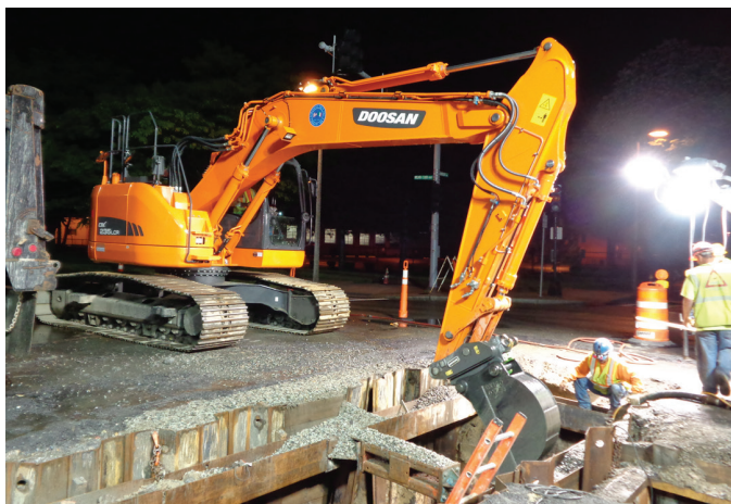
One major project currently being worked on by AD&S is BWSC Contract 11-309-009 Dudley Square Sewer Separation Project
