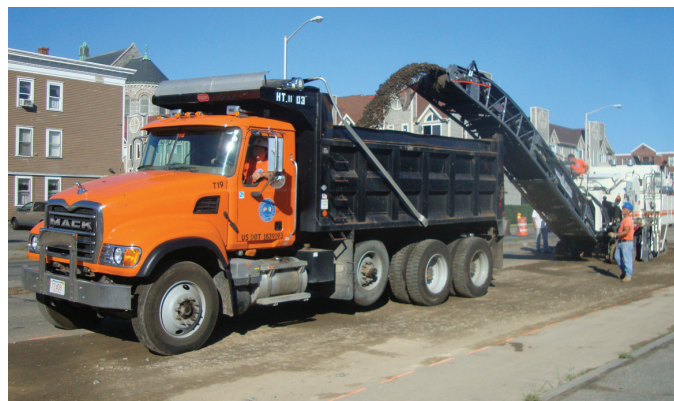
Lowell Regional Wastewater Utility – Cabot Street Area Sewer Separation Contract 10-01 Father Morissette Boulevard (2010)
