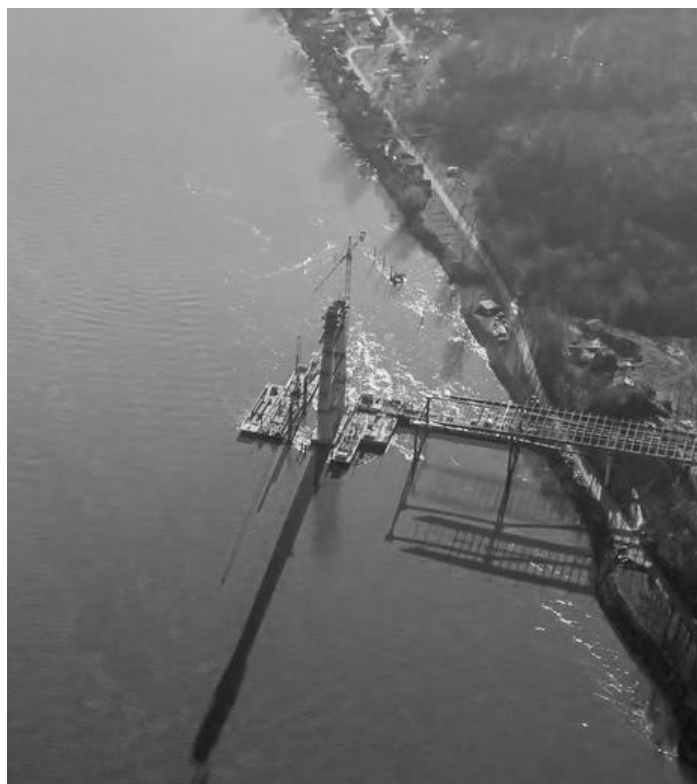
The Lewis and Clark Bridge connected I-265 through Southern Indiana to the East End of Louisville, placing Utica along a major transit corridor.
