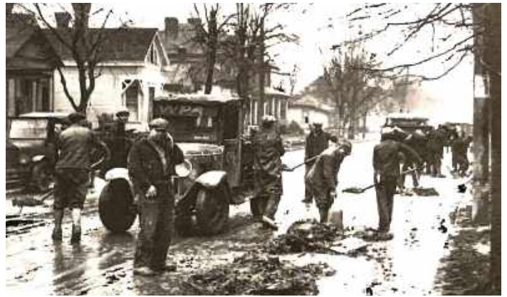
WPA workers clear debris from Maple Street in Jeffersonville after the 1937 flood. Courtesy of the Jeffersonville Township Public Library.
