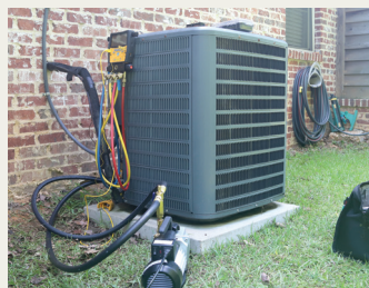
Pre-season HVAC tune ups
