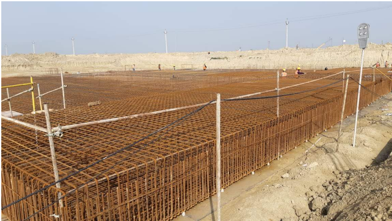
Civil Works of BOP at 2x660MW Jawaharpur Thermal Power Plant. District:-Etah, Uttar Pradesh
