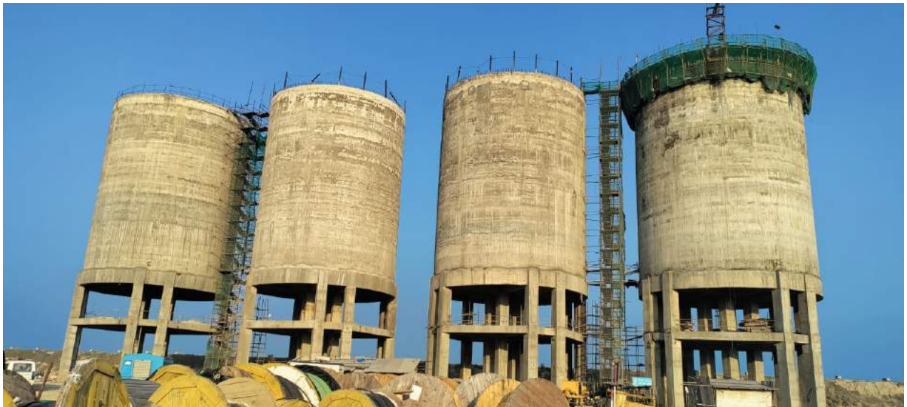
Four nos. Ash Silo's at 2x660MW Jawaharpur Thermal Power Plant. District:-Etah, Uttar Pradesh
