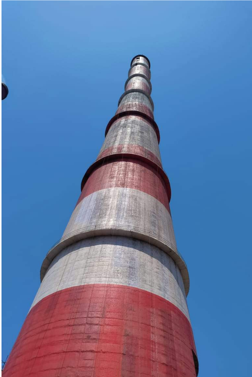
275 Mtrs high RCC Chimney at Unit#2 3x660MW NTPC North Karanpura, Distt:- Chatra (Jharkhand).
