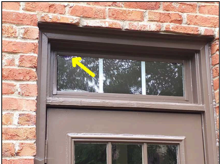
Warped/bulging seals noted at window above deck door
