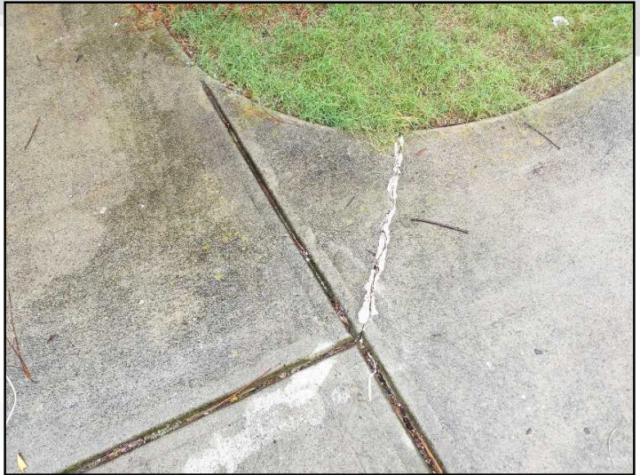
Typical cracking noted in driveway
