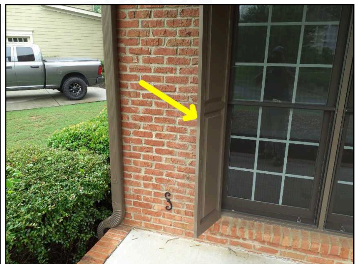
Correct multiple detached exterior window shutters
