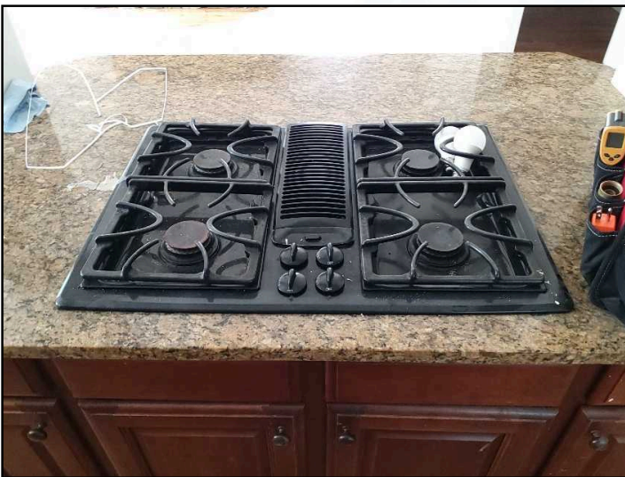
Multiple controls at the kitchen gas cooktop are not operational. Recommend repair or replacement
