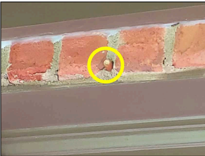
Drainage weep channels in exterior brick are clogged sporadic around home.
