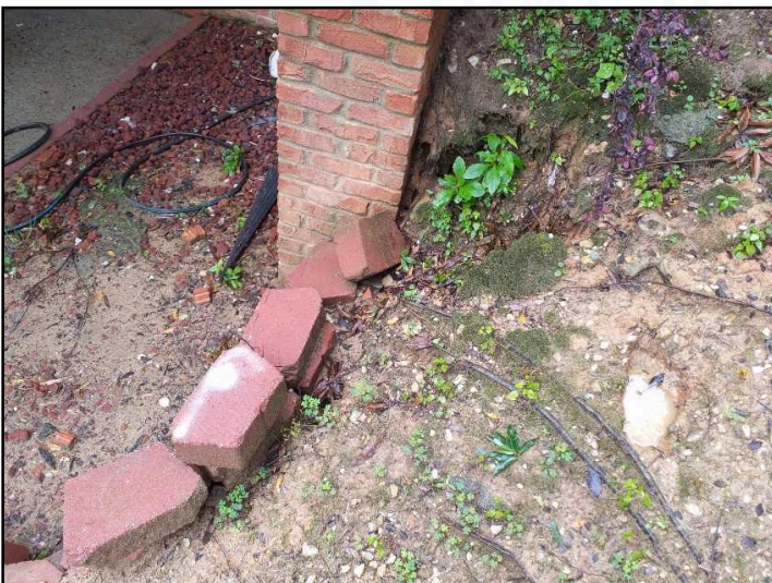
Concrete block portion of retaining wall at back left side of Home needs replacement
