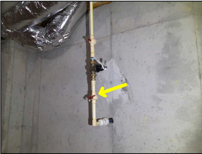
Main water shut off noted at the front basement wall
