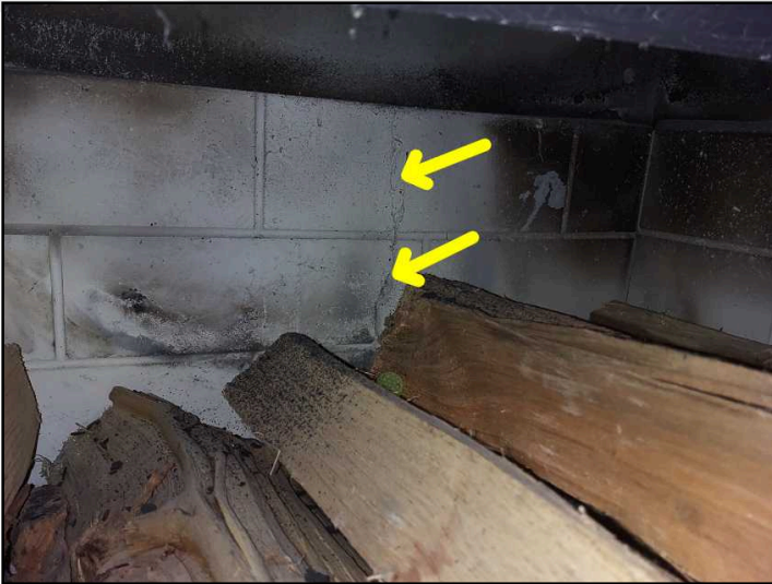
Minor cracking and deterioration on back fire brick. Have a chimney sweep examine and repair as needed for safe use.
