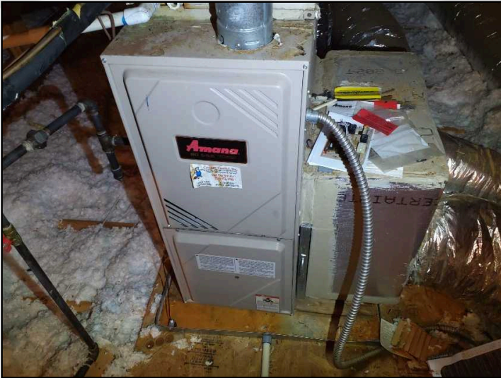
Gas furnace in attic Amana 2003 unit is beyond its normal life expectancy
