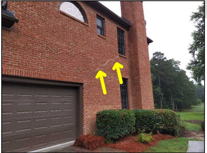
A large step crack at the right exterior brick veneer has been sealed. Inquire with seller for any available documentation on repair, continue monitoring and seek further evaluation by Brick Mason as desired
