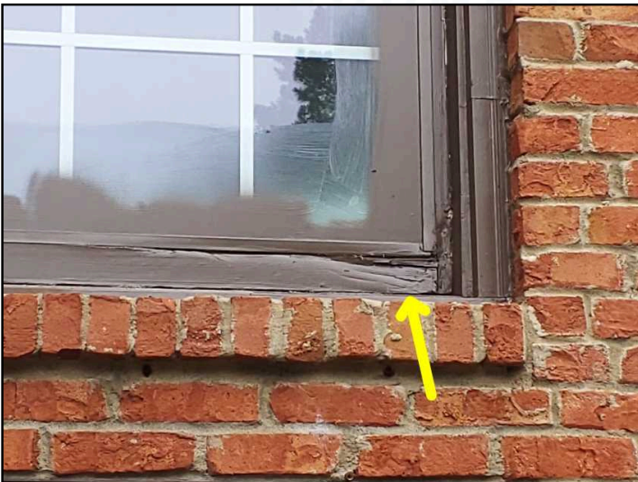
Replacement needed at extensive water damage to window frames above back deck
