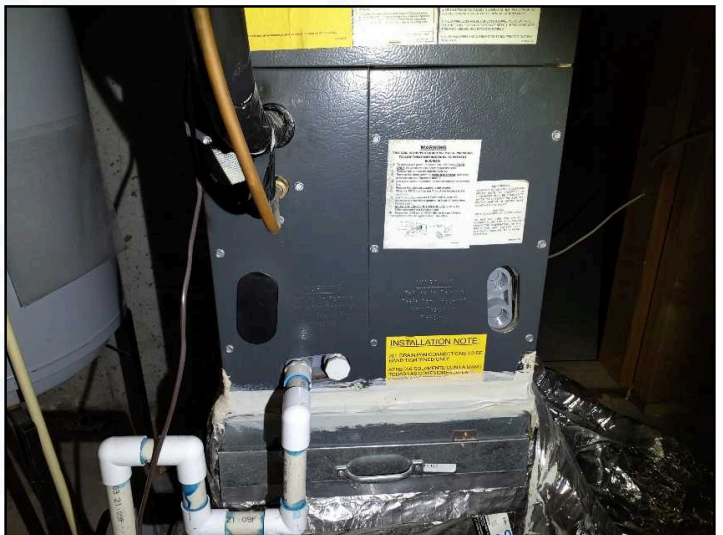
Basement electric HVAC system 2004 Goodman unit is beyond its normal life expectancy
