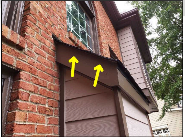
There is no drip edge flashing present where the roof shingles end to cover the connection at the lateral rake boards.
