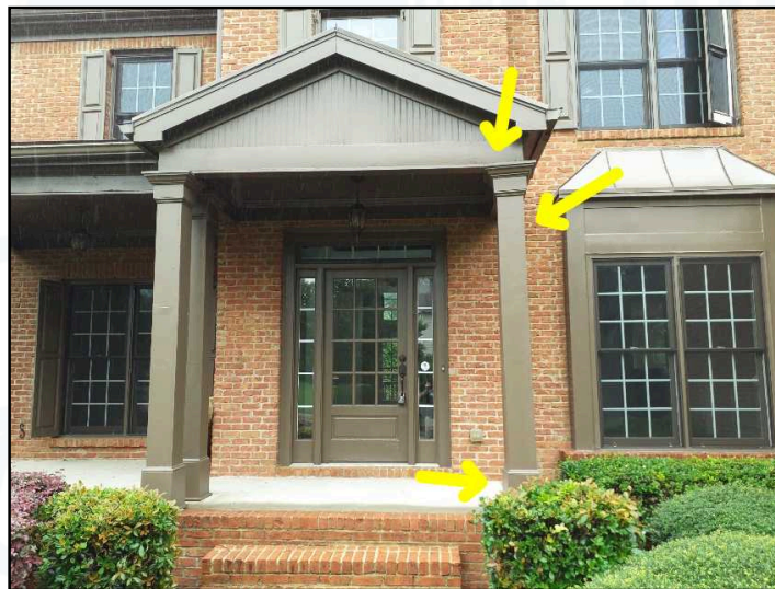
Decorative housing at front right porch support post is slightly warped or twisted. Unable to determine condition of structural member inside housing. Recommend further evaluation and correction as needed
