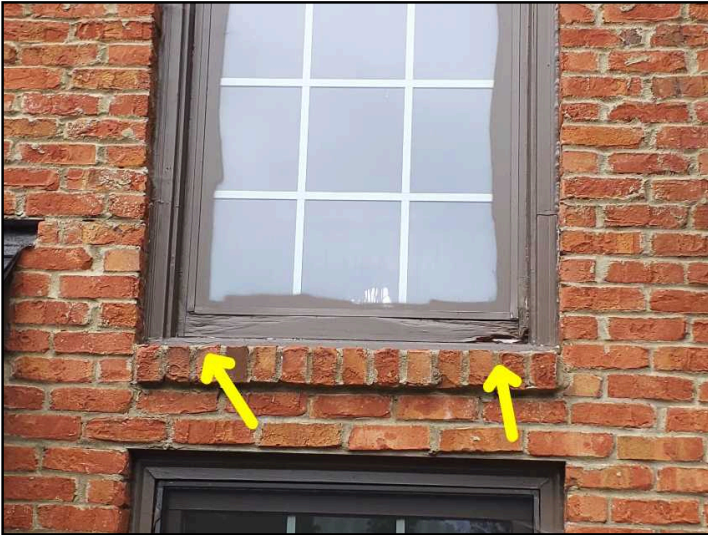
Replacement needed at extensive water damage to window frames above back deck
