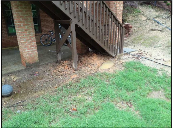
Landscaper needed for poor drainage, bare soil and erosion
