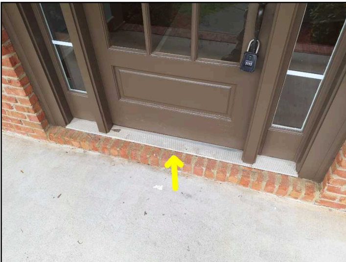
Caulk thresholds under exterior doors
