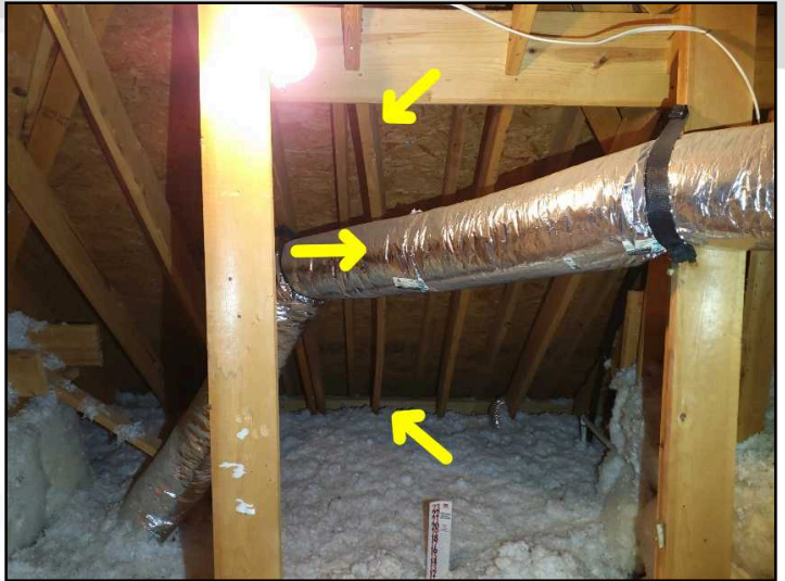
Lateral roof support framing in attic space between edge of roof line and entrance ladder is Warped and bent. Recommend repair or replacement by qualified contractor
