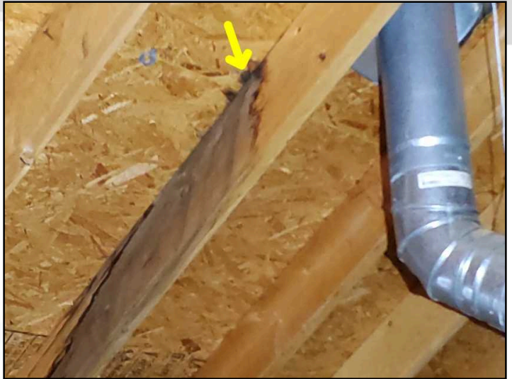
Evidence of water intrusion at exhaust pipe flashing Fastener with staining in attic space below. Recommend correction by qualified roofer
