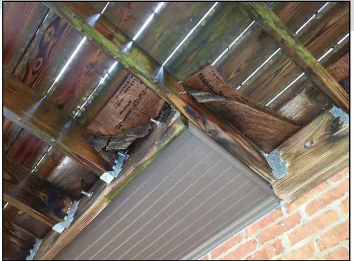
There is no visible flashing where deck meets house. The joint between the deck and the house should be flashed to prevent water penetration where the deck is bolted to the home.
