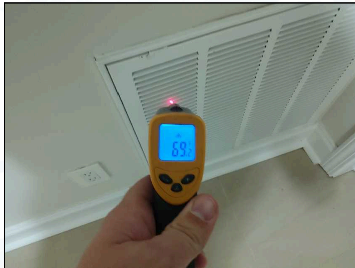
There was a 13 degree temperature differential when the air conditioning was tested at the basement level.
