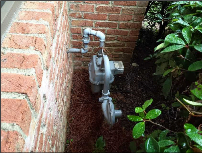
Gas meter at the right exterior side
