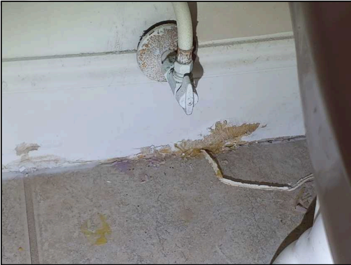
Water damage at baseboard behind main level toilet from leak at toilet tank above
