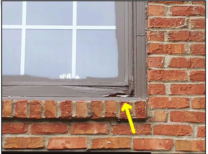
Replacement needed at extensive water damage to window frames above back deck
