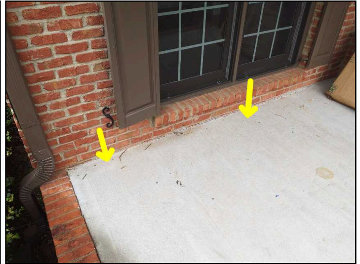
Seal gap where house and porch meet to prevent water from entering structure
