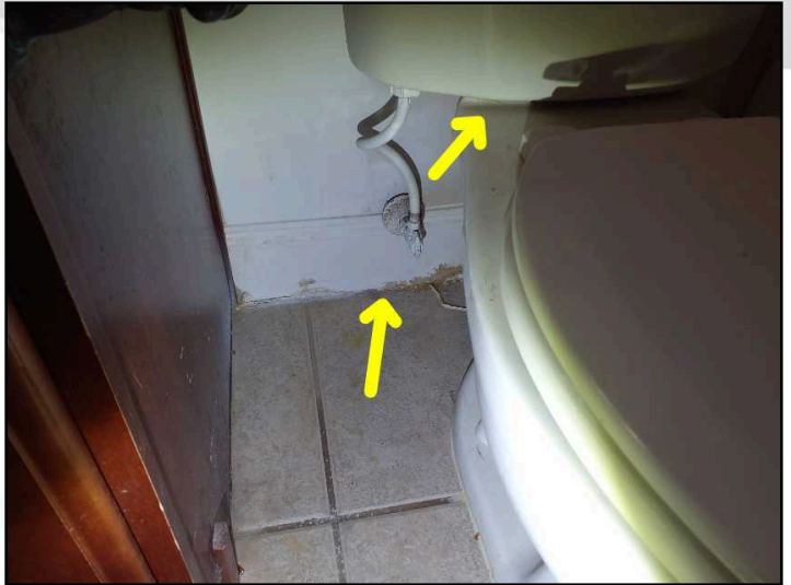
Water damage at baseboard behind main level toilet from leak at toilet tank above
