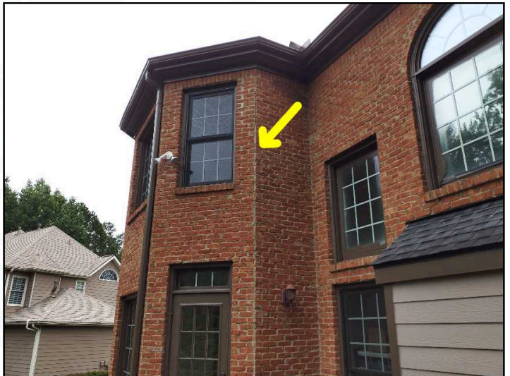
Repair crack in exterior brick veneer above deck door
