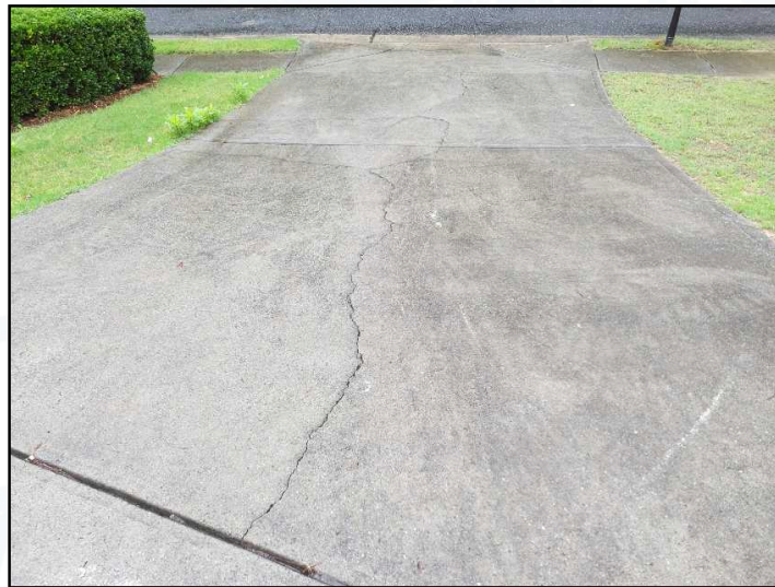
Typical cracking noted in driveway
