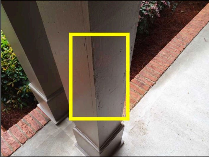
Patched water damage at exterior trim
