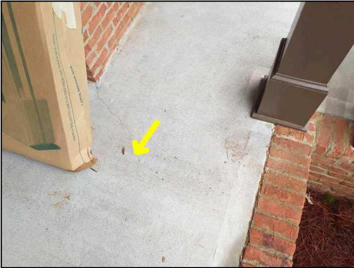
Monitor typical cracking at concrete front porch slab
