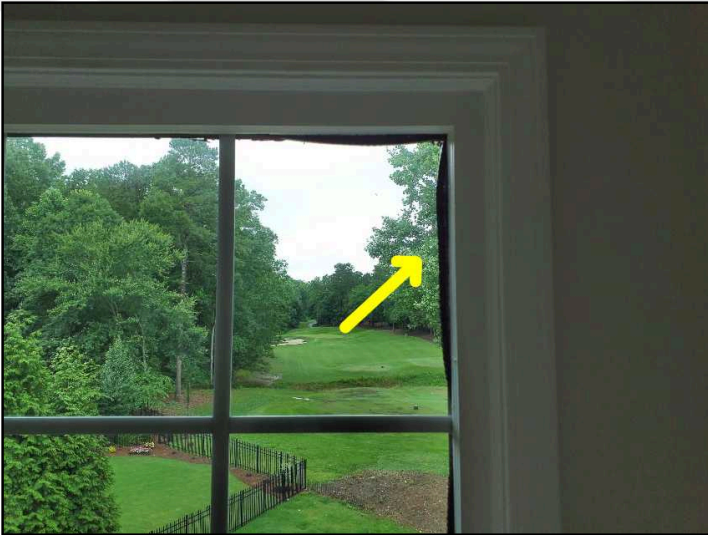
Warped/bulging seals noted at window in master bedroom
