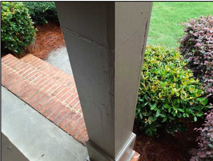
Patched water damage at exterior trim
