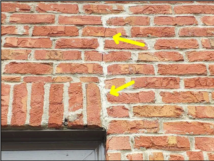
A vertical crack at the right exterior brick veneer above the garage has been sealed. Inquire with seller for any available documentation on repair, continue monitoring and seek further evaluation by Brick Mason as desired
