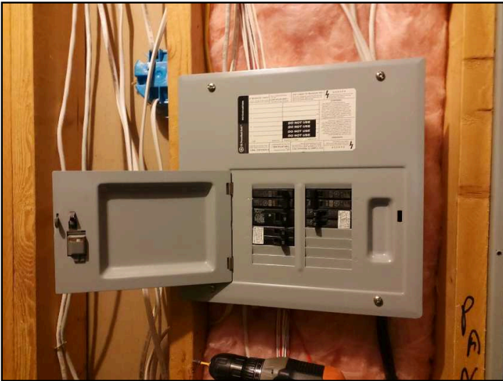
Sub panel located at the basement
