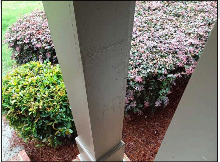
Patched water damage at exterior trim
