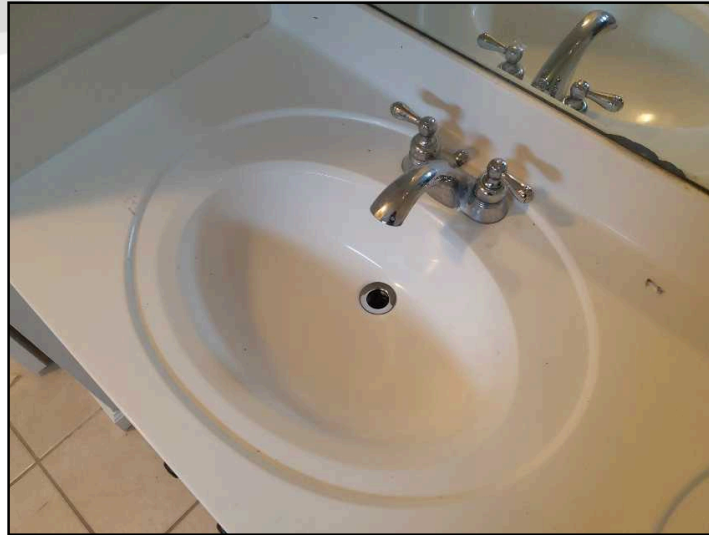
Non-functioning drain stopper noted in the Jack N Jill Bath
