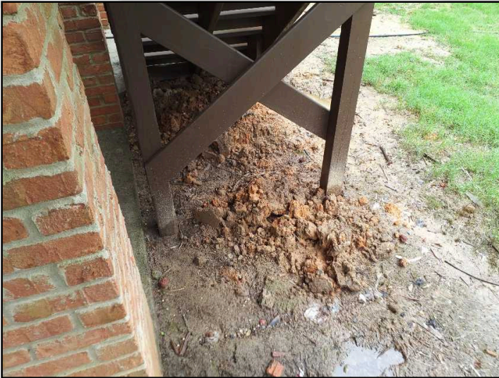
Wood deck support posts/framing should not be in direct contact with soil and will increase rate of deterioration and increase potential for movement/wood destroying organism activity
