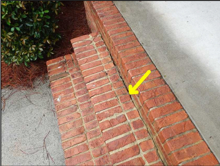
The front exterior brick steps have settled leaving a small Gap at connection to porch above. Recommend repair and continued monitoring
