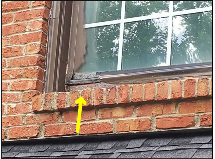
Replacement needed at extensive water damage to window frames above back deck
