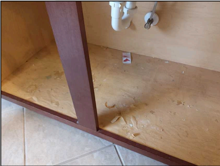
Water stains/damage at vanity cabinet
