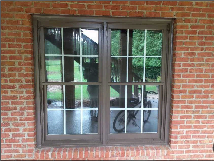
Missing window screens observed. Have screens installed for proper ventilation.
