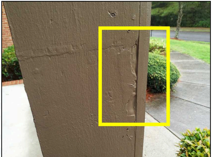
Patched water damage at exterior trim
