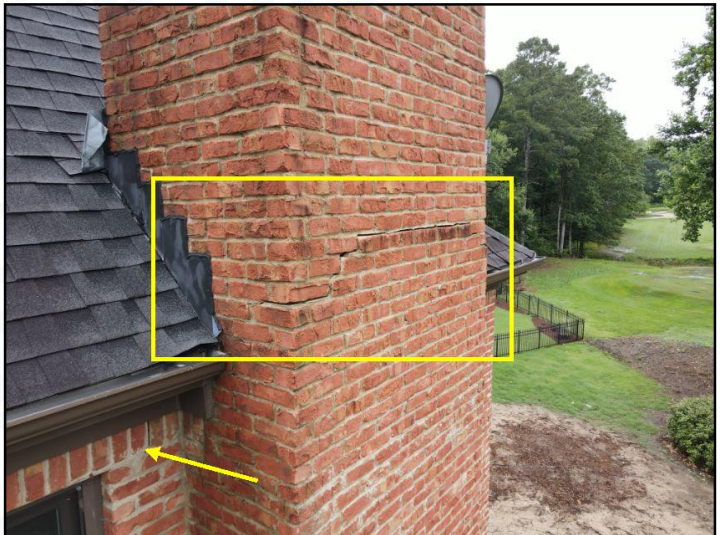
The chimney is leaning towards the home above the roof line. Horizontal cracks are noted in the siding at the roof line. Have a qualified contractor or structural engineer examine the chimney and determine if repairs are needed to correct the movement or stabilize it in its current condition and seal any cracks in the siding.
