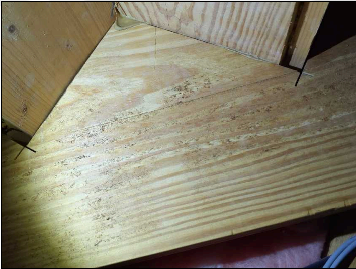
The inspector observed a substance resembling microbial fungal growth partially covering the sub floor structure and framing members in the basement below the staircase.
