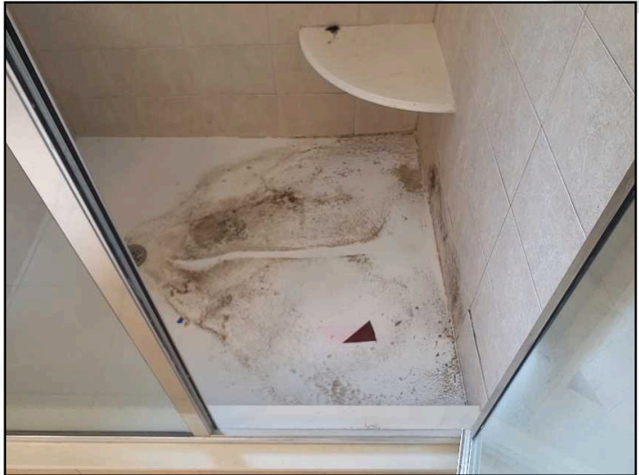
Evidence of leak at master bathroom shower head resulting in mold like growth inside shower stall. Recommend testing to determine type of growth present which Serenity Home Inspections can perform and correction of leak and treatment of growth
