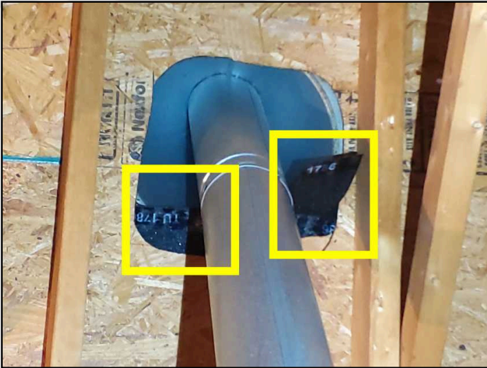
The exhaust vent pipe has inadequate clearance to in the attic space which is a safety concern. The vent is should have at least a 1" clearance from the insulation/felt paper. Have corrections made.
