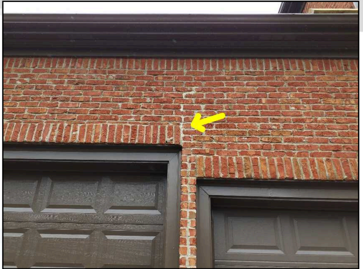
A vertical crack at the right exterior brick veneer above the garage has been sealed. Inquire with seller for any available documentation on repair, continue monitoring and seek further evaluation by Brick Mason as desired
