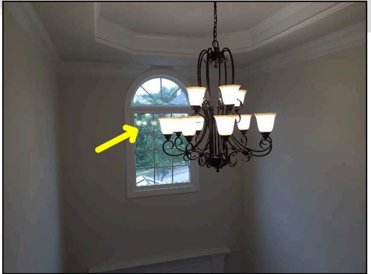
Warped/bulging seals noted at window above front door in foyer
