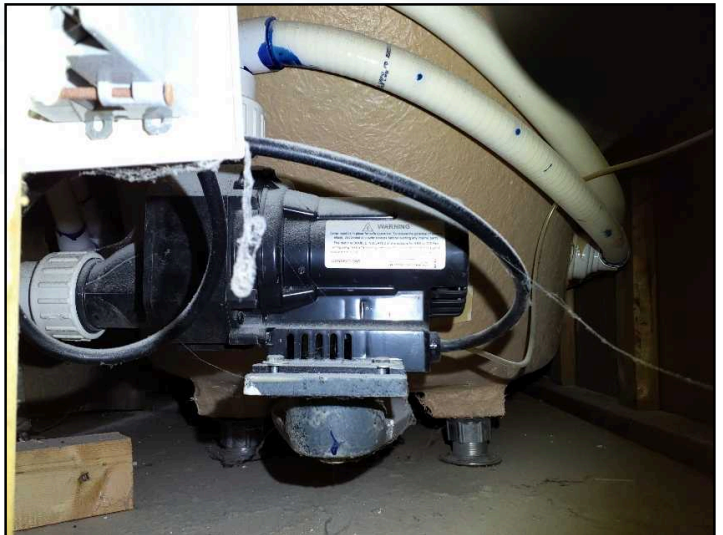
Jetted tub motor
