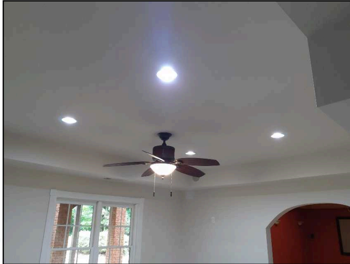
Flickering observed at recessed lighting in basement surrounding ceiling fan. Recommend further evaluation for cause and correction
