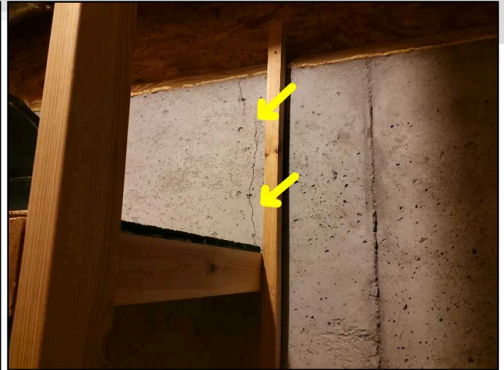
Common cracks observed. These should be sealed as needed and monitored for any future leaks or movement.
