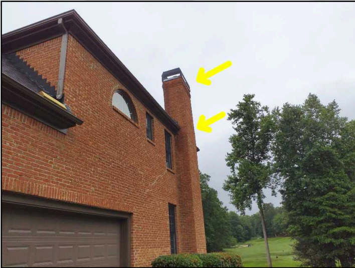
Horizontal and step cracking observed at exterior portion of chimney in brick veneer on right side of home near connection to gutter. Recommend further evaluation by qualified contractor to ensure structure of Chimney is not leaning or compromised and repair brick to prevent water intrusion
