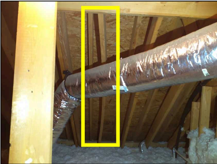
Lateral roof support framing in attic space between edge of roof line and entrance ladder is Warped and bent. Recommend repair or replacement by qualified contractor
