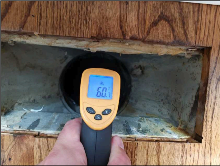
There was a 12 degree temperature differential when the air conditioning was tested at the main floor level.
