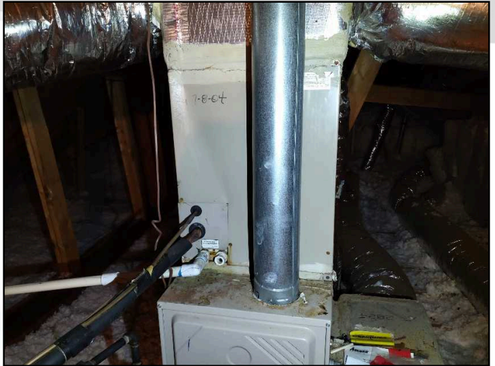
Evaporator coil portion in attic space 2003 unit is beyond its normal life expectancy
