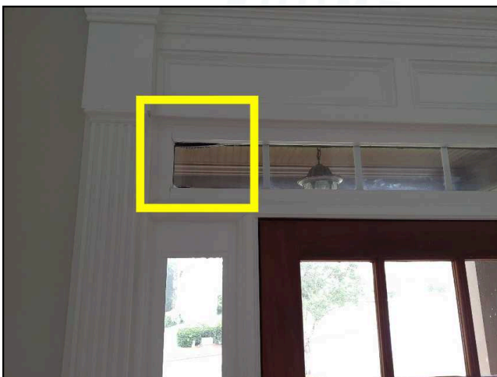
Bulging seals at window above front door
