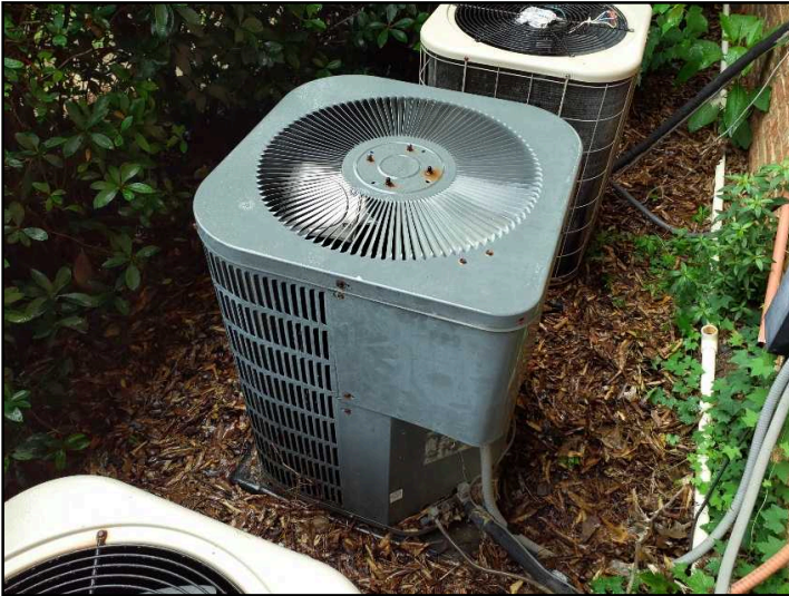
Center exterior Goodman AC unit
