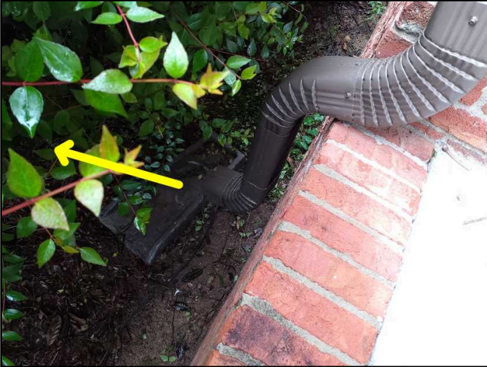
Reconnect extension to gutter down spout
