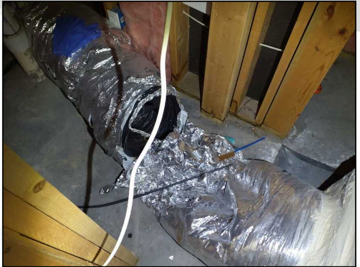
The supply duct for the basement HVAC system is broken and attached
