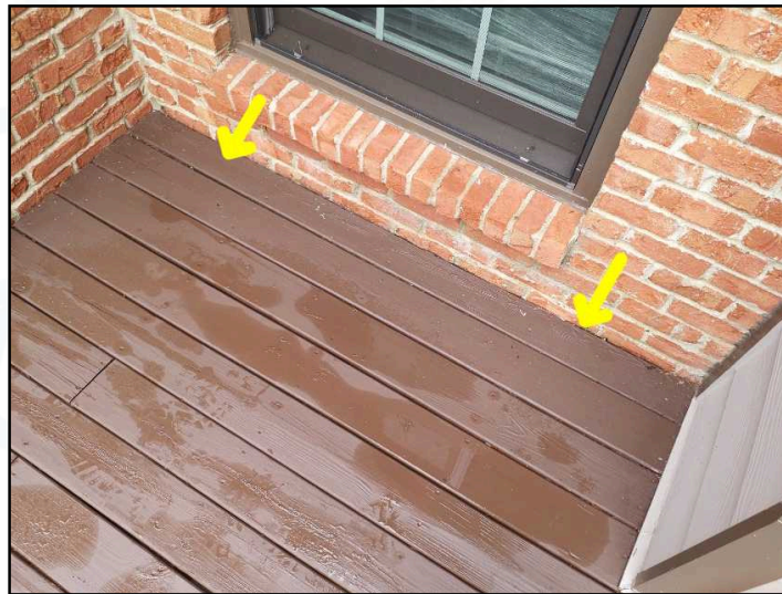
There is no visible flashing where deck meets house. The joint between the deck and the house should be flashed to prevent water penetration where the deck is bolted to the home.
