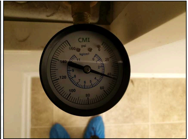
Water pressure measured 40-45 pounds per square inch (psi) at the time of the inspection. Acceptable water pressure is between 40 and 80 psi.
