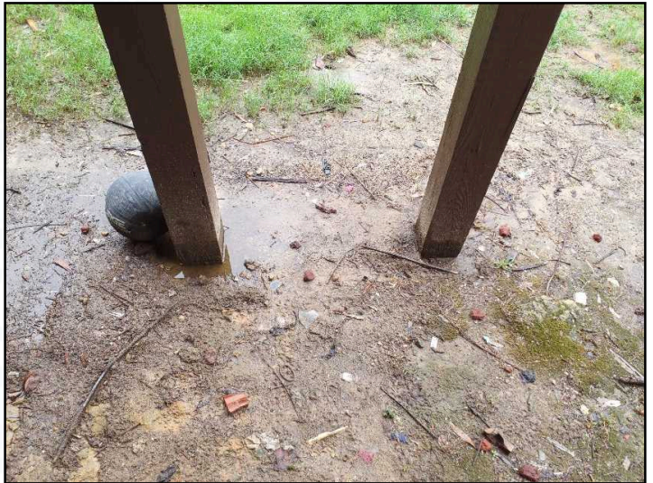
Wood deck support posts/framing should not be in direct contact with soil and will increase rate of deterioration and increase potential for movement/wood destroying organism activity
