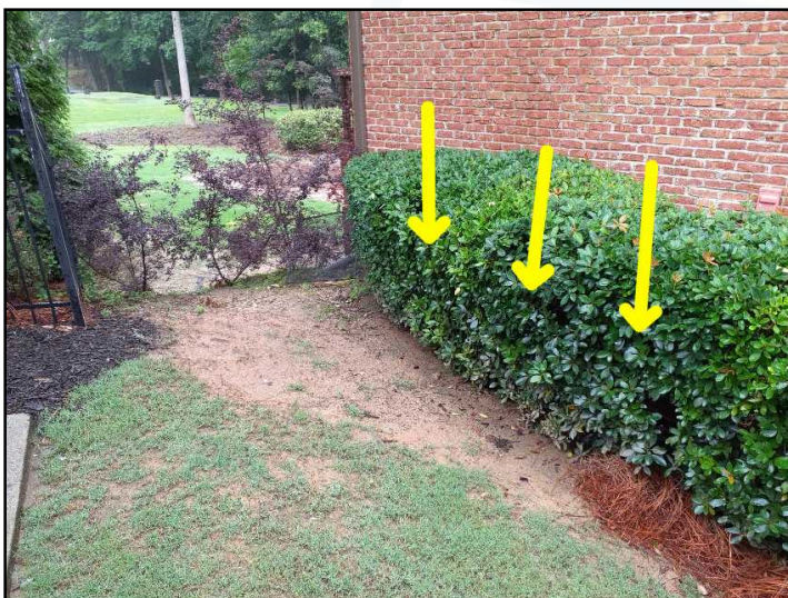
Incorrect soil slope at back left corner
