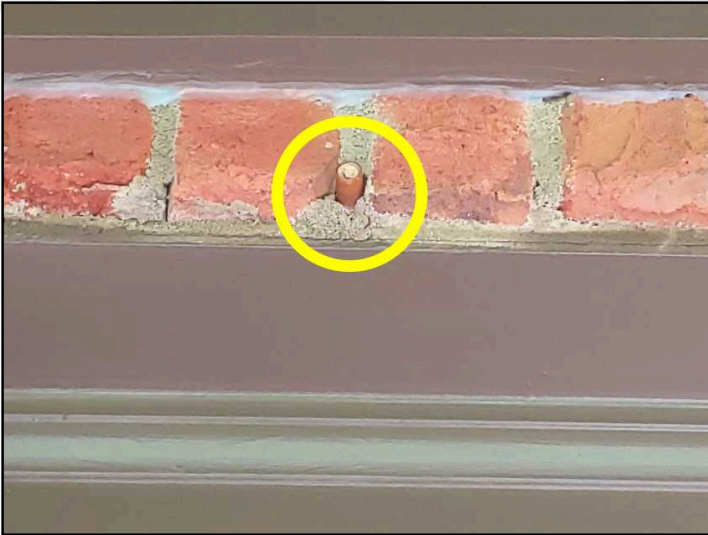
Drainage weep channels in exterior brick are clogged sporadic around home.
