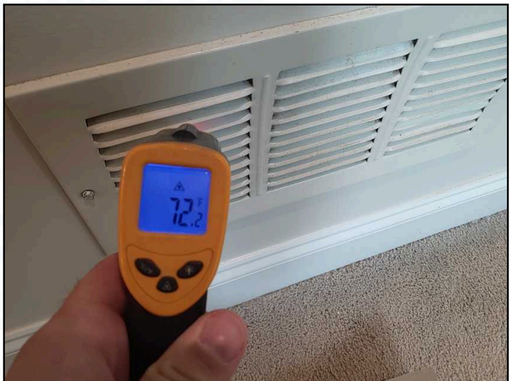
There was a 12 degree temperature differential when the air conditioning was tested at the main floor level.
