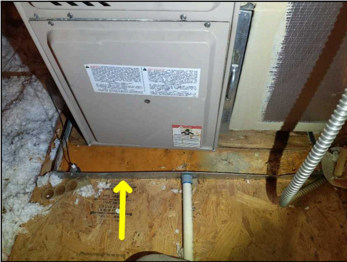
Rust is noted in the overflow pan under the attic unit. Have an HVAC contractor review condensate system to determine reason for rust and correct as needed.
