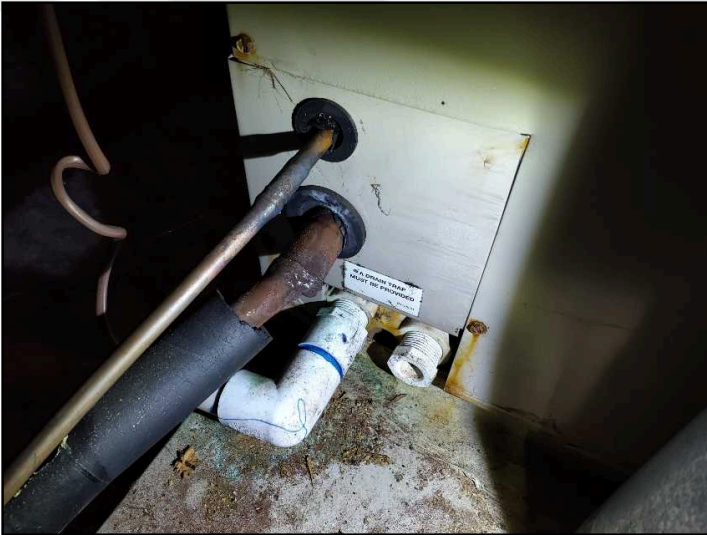
Seal and insulate the copper AC lines where they meet the coils at the top or side of the furnace. Conditioned air is being lost to the space around and condensation is dripping from the copper lines.
