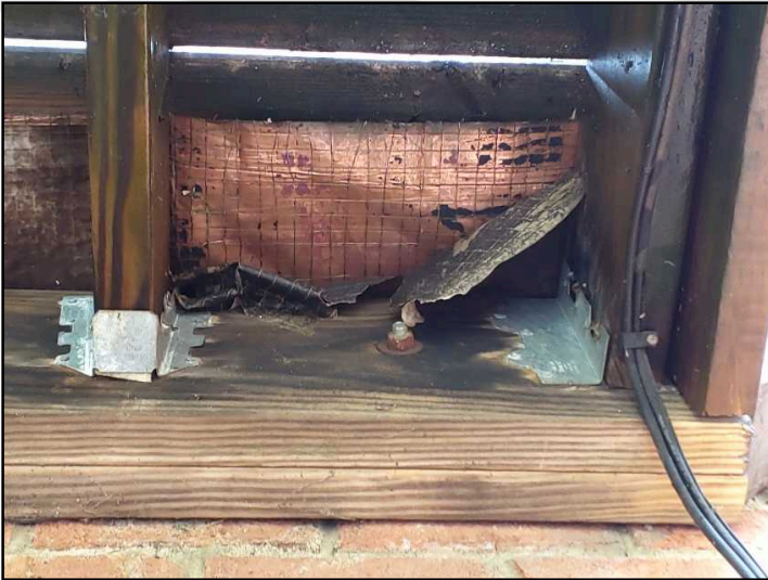
There is no visible flashing where deck meets house. The joint between the deck and the house should be flashed to prevent water penetration where the deck is bolted to the home.
