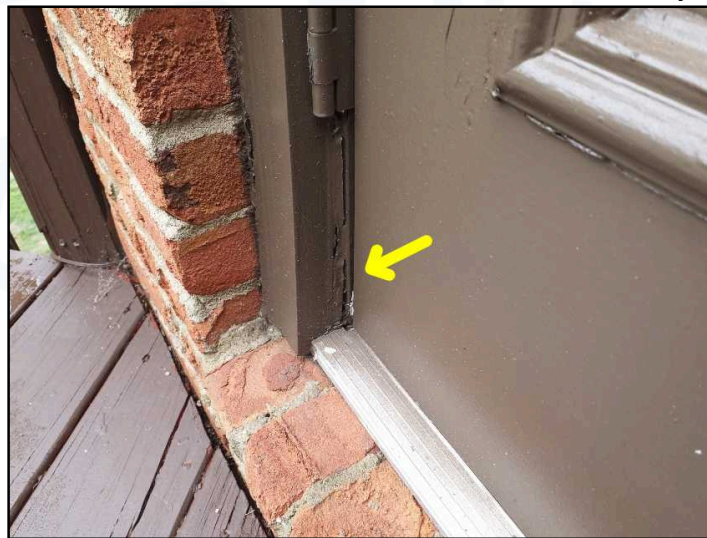
Trim is separating at back deck exterior door frame and may allow rain intrusion
