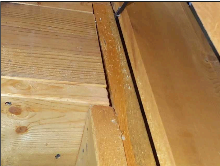
The inspector observed a substance resembling microbial fungal growth partially covering the sub floor structure and framing members in the basement below the staircase.
