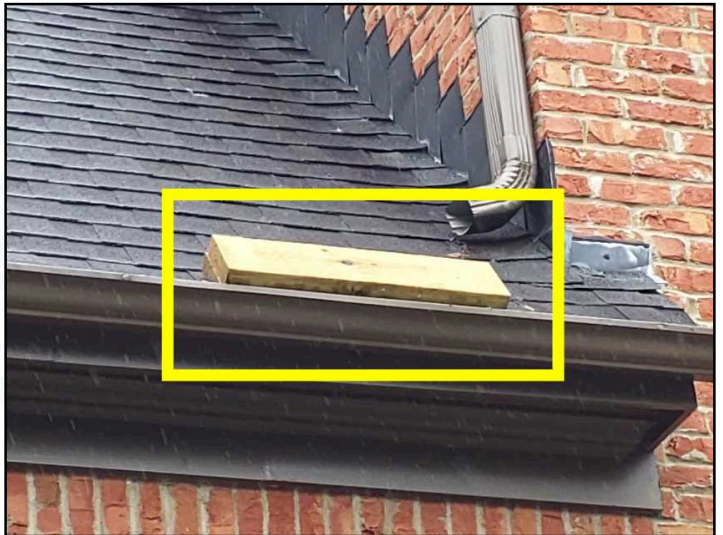
Remove wood debris on roof above garage door and install proper flashing if needed
