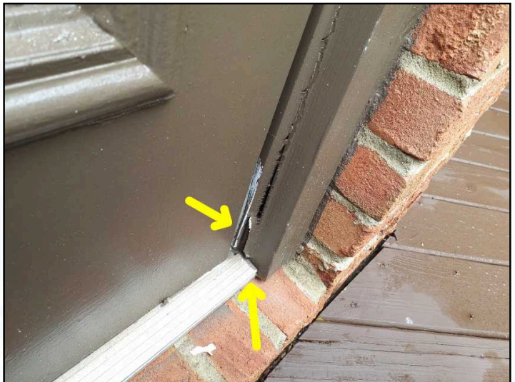
Trim is separating at back deck exterior door frame and may allow rain intrusion
