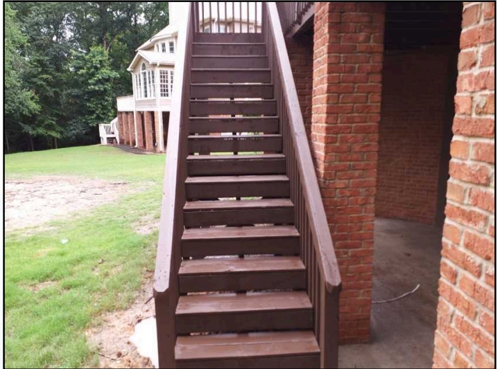
The handrail is not graspable. Deck/porch stairs require a graspable, continuous and smooth handrail for safety. A 2x4 or 2x6 board is not an acceptable hand rail.
