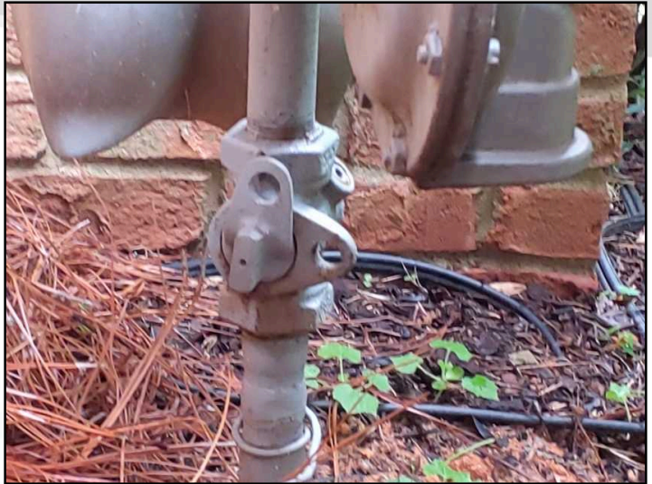
Gas meter at the right exterior side
