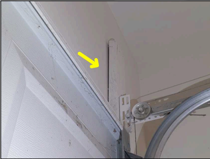
Loose framing noted at garage door(s)
