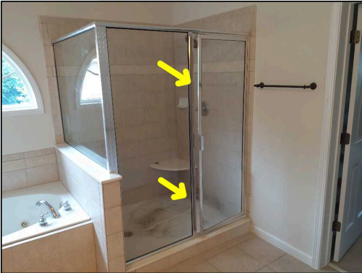
the master bathroom shower stall door is loose, misaligned or sticking making proper operation more difficult. Repair or replace as needed.
