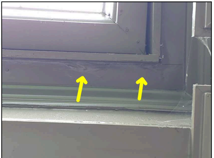
Patched water damage at exterior trim
