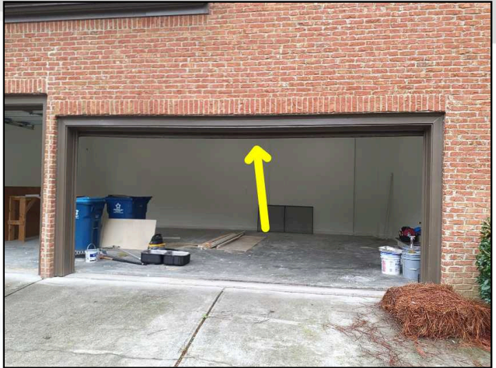
The two car garage overhead door stops slightly short of fully opening. Recommend adjustment
