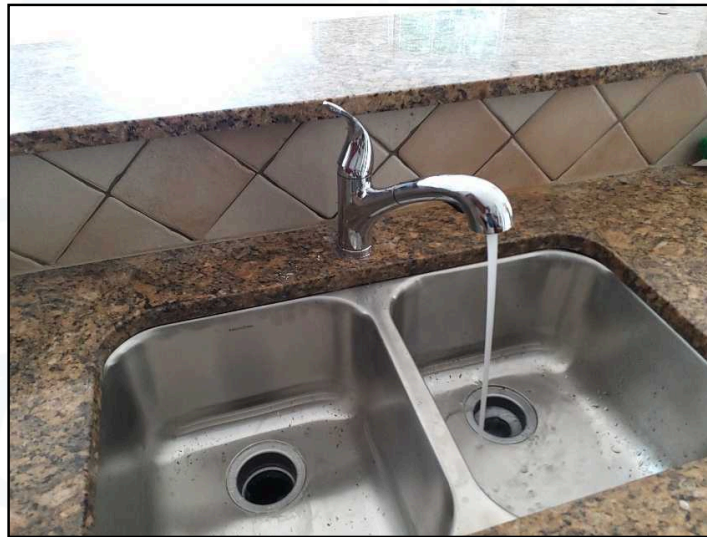
There is no cold water pressure at the kitchen sink faucet
