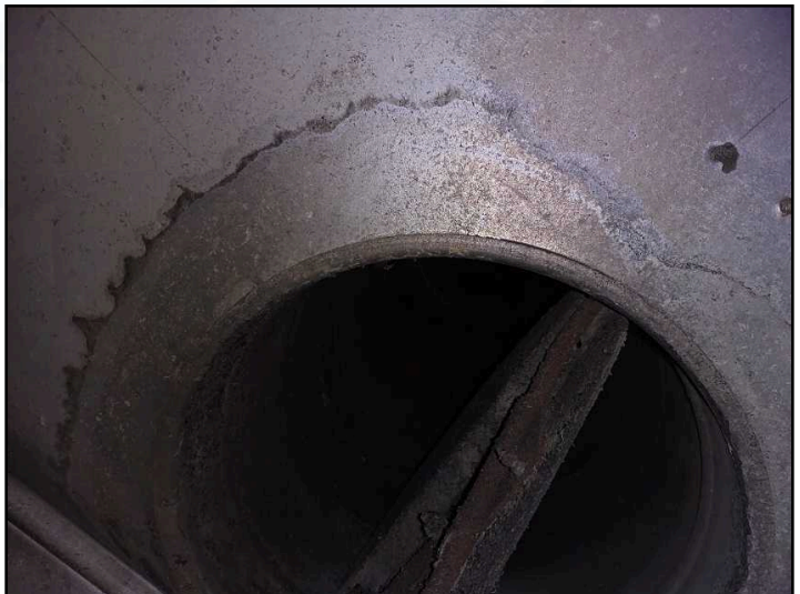
Fireplace damper image
