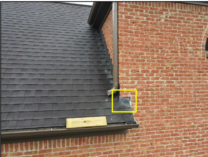
Horizontal apron flashing connecting roof shingles to brick veneer above garage Overhead Doors near base of upper downspout has separated and may allow rain intrusion into roof cavity below
