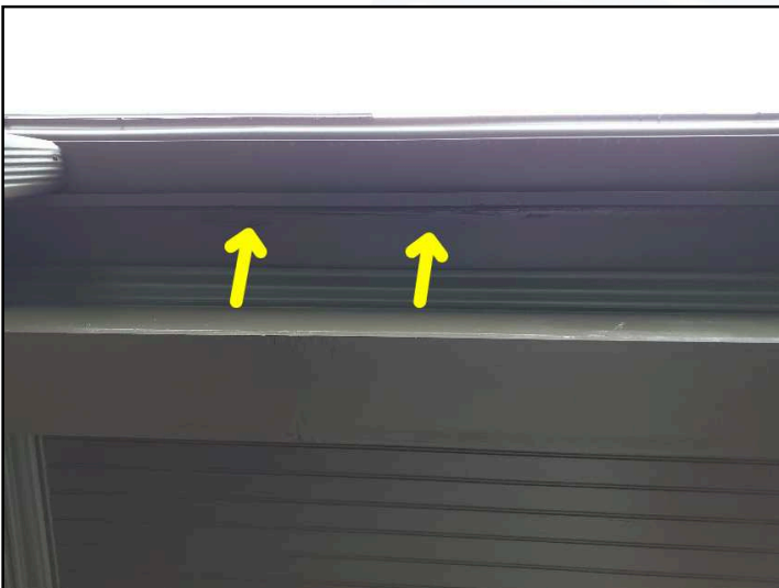
Patched water damage at exterior trim
