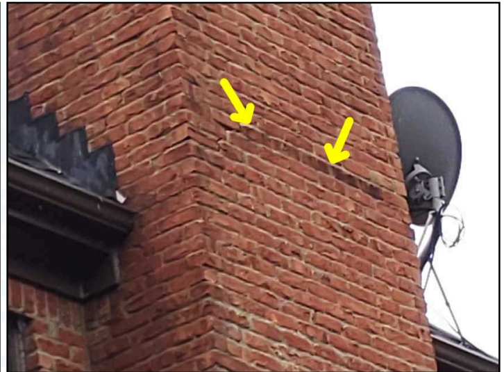
Horizontal and step cracking observed at exterior portion of chimney in brick veneer on right side of home near connection to gutter. Recommend further evaluation by qualified contractor to ensure structure of Chimney is not leaning or compromised and repair brick to prevent water intrusion
