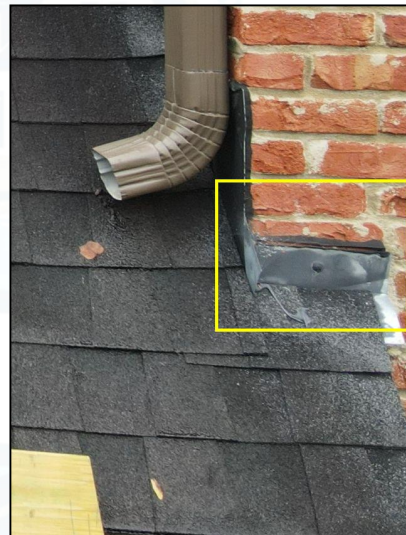
Horizontal apron flashing connecting roof shingles to brick veneer above garage Overhead Doors near base of upper downspout has separated and may allow rain intrusion into roof cavity below
