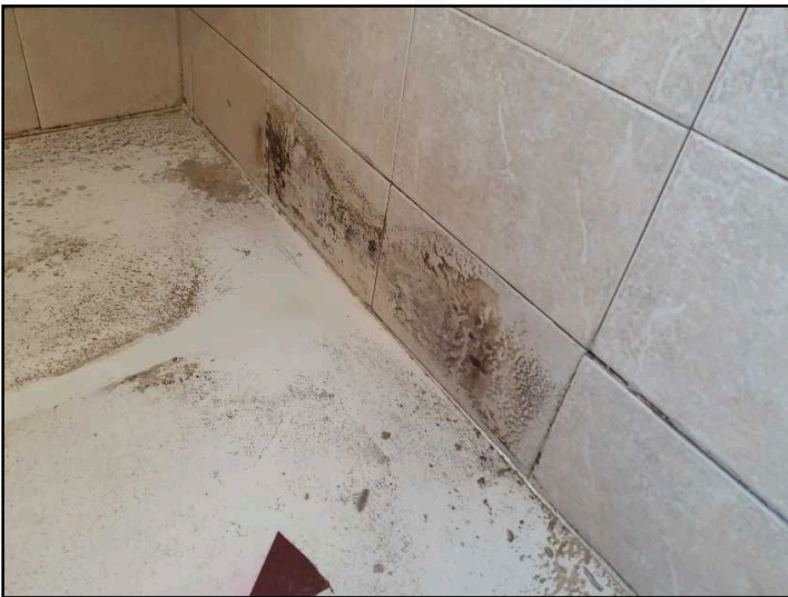
Evidence of leak at master bathroom shower head resulting in mold like growth inside shower stall. Recommend testing to determine type of growth present which Serenity Home Inspections can perform and correction of leak and treatment of growth
