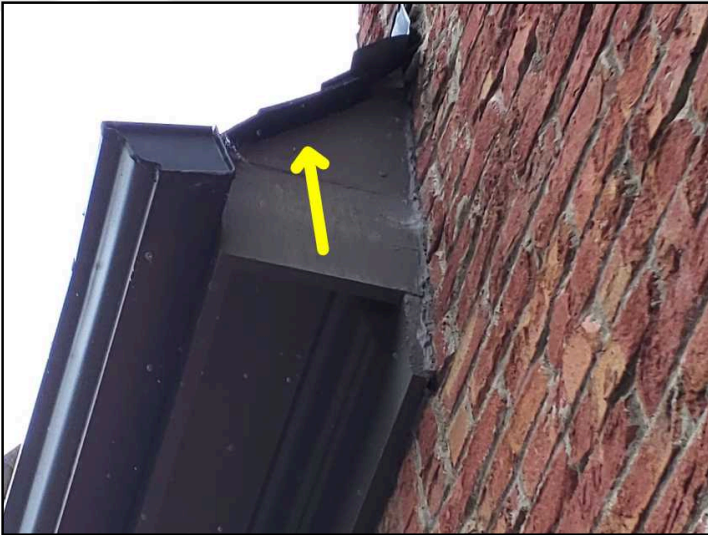
There is no drip edge flashing present where the roof shingles end to cover the connection at the lateral rake boards.
