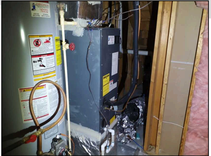
Basement electric HVAC system 2004 Goodman unit is beyond its normal life expectancy
