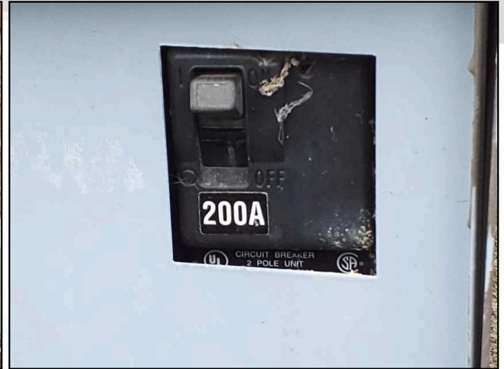
Electric meter and 200 amp shut off at the right exterior side
