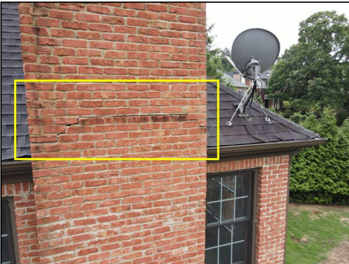
The chimney is leaning towards the home above the roof line. Horizontal cracks are noted in the siding at the roof line. Have a qualified contractor or structural engineer examine the chimney and determine if repairs are needed to correct the movement or stabilize it in its current condition and seal any cracks in the siding.
