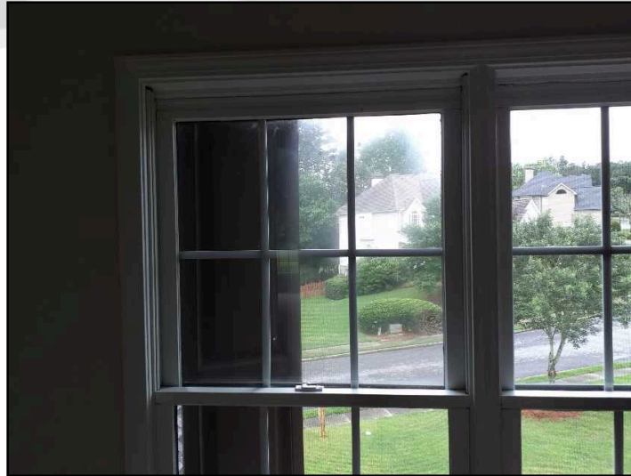
Thermal seal failure observed at window in the Upper Front right guest bedroom
