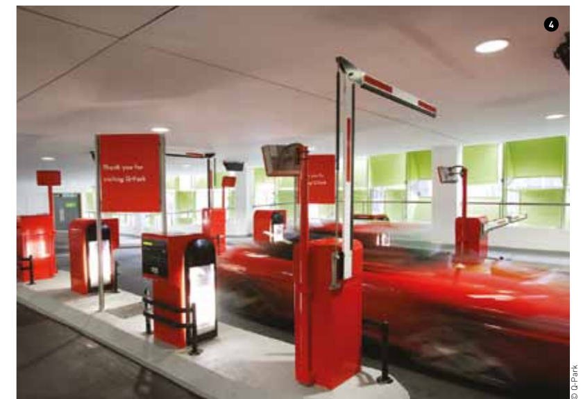
3 Q-Park, Sheffield, England Energy savings are instant, with luminaires being active only when needed.
