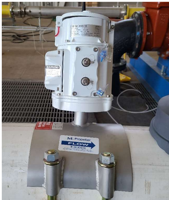
Figure 16. McCrometer FlowConnect telemetry unit and flow meter
