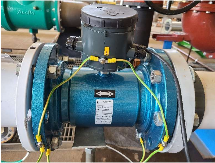
Figure 43. Bermad Model MUT2200EL flowmeter with telemetry
