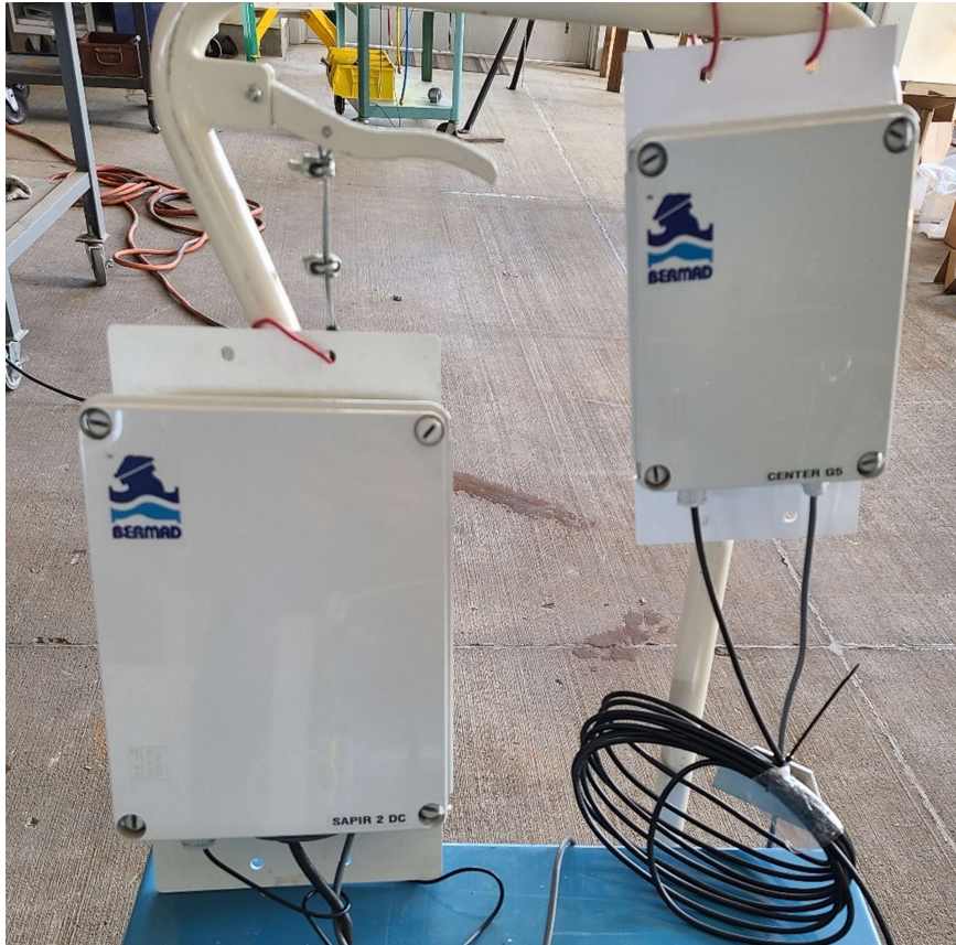
Figure 44. Bermad telemetry datalogger and cellular unit
