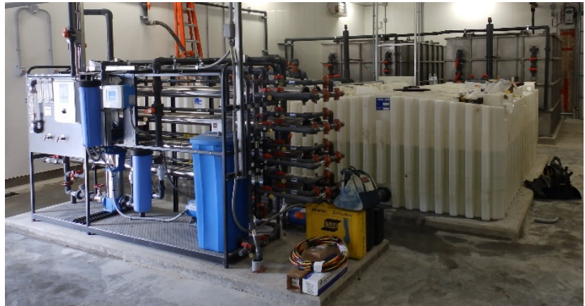
Filtered water pumped into nanofiltration system (Similar to Island Lake)
