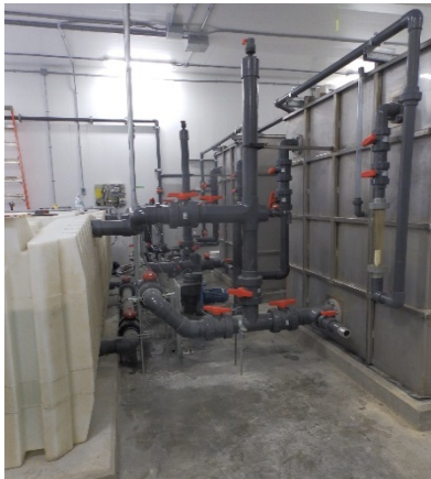
Filters producing to storage tank
