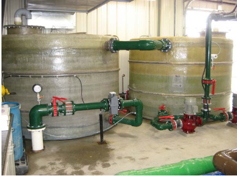
Figure 9. Two contact tanks used to ensure formation of micro-flocs and transfer pumps that take the water to the filters.
