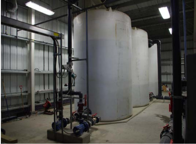
Figure 14. Contact tanks and transfer pumps.
