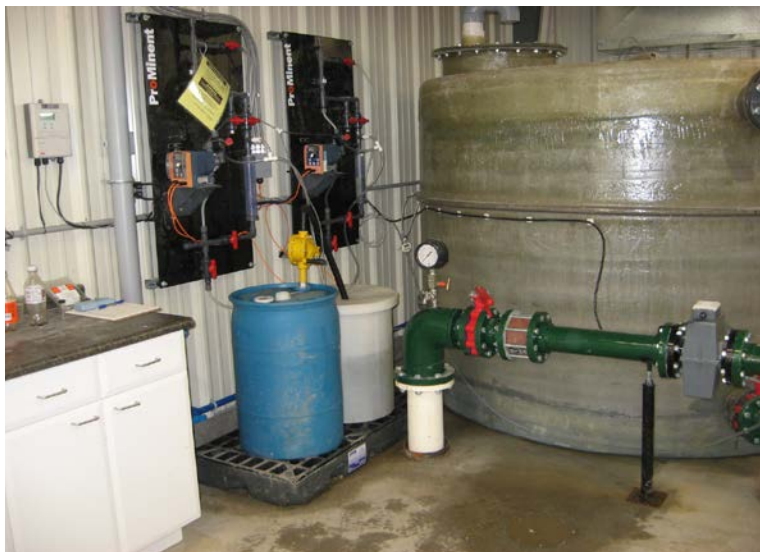
Figure 8. Inlet from well, flow meter and chlorine dosing equipment. (Note lab bench and equipment at left.)
