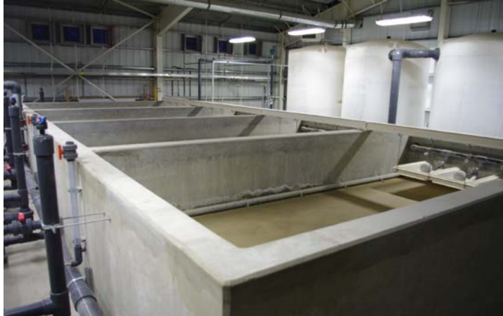
Figure 13. Interior view of water treatment plant.
