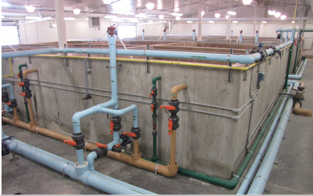
Figure 18. Interior of WTP3.
