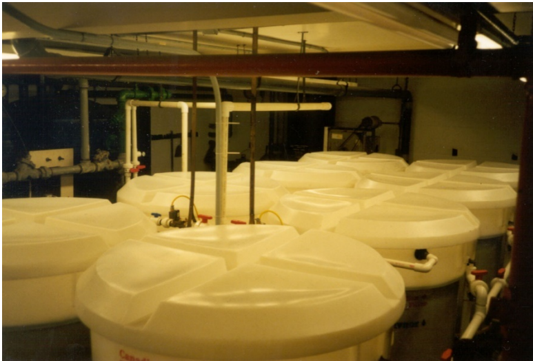
8 x 1000 Lph polyethylene PF filters followed by GAC and chlorine disinfection.
