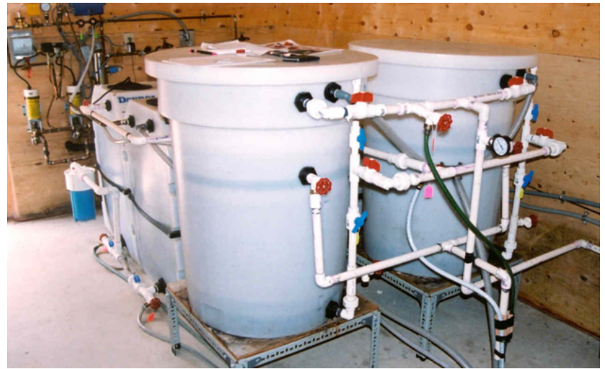
2 x 180 Lph BF polyethylene filters followed by UV disinfection.
