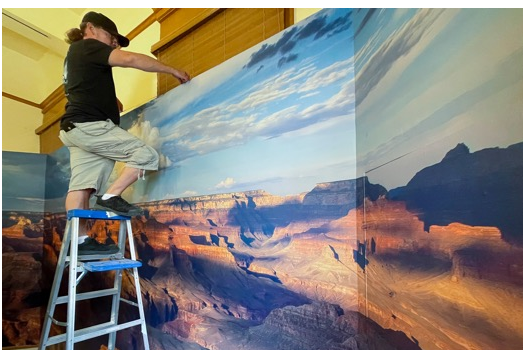
A worker installs the Grand Canyon north rim mural. The 9' by 27' photograph was made by professional photographer Dianne Dietrich-Leis.
