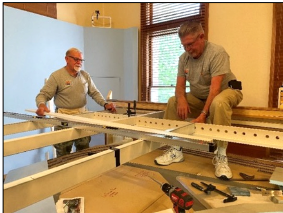
On March 29, 2022, Ray and Ken start adding the supports for the upper plywood for the Grand Canyon South Rim. Don Stewart photo
