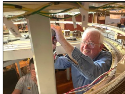
Jesse Poole, right, and Ken Nelson install one of the motorized lift sections in the Helix below Williams.
