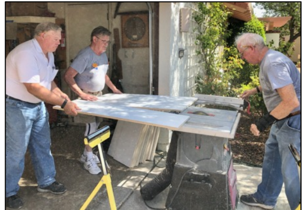
Don Stewart, Ken Nelson and Jesse Poole cut plywood for the custom rolling stock cabinets.
