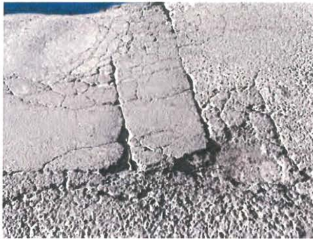
Photo 2.6.1-1. Cracked pavement over traffic signal detector.
