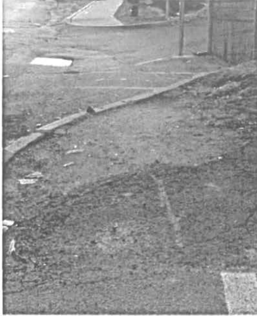
Photo 2.6.1-5 Asphalt sidewalk not complete to driveway and no accessible ramp.
