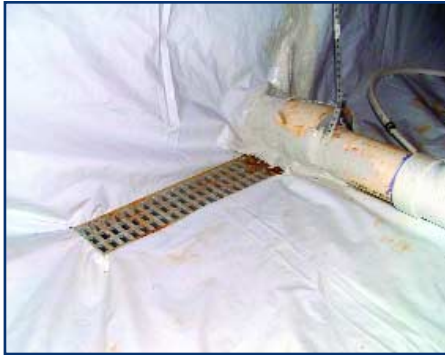
The finished ground vapor retarder is sealed directly to the drain opening.
