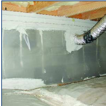
Vapor retarder material is attached with a furring strip three inches (76 mm) below the top of the masonry wall and sealed to the wall with mastic. The wall vapor retarder material is sealed to the ground vapor retarder to form a continuous liner. Penetrations, like the dryer vent in the photo, are completely air sealed. The top of the masonry wall and the front edge of the sill plate have been painted white with mastic to improve inspectability by pest management professionals.
