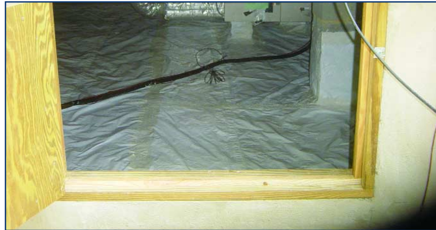
The entrance to this closed crawl space is elevated well above exterior grade, reducing the likelihood of water entry in heavy rains or minor flooding. Photo credit: Indoor Environmental Systems.
