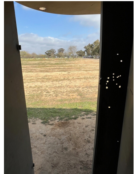
Bullet holes in the wall at the site of the Nova music festival. These bomb shelters were used by attendees to try and hide but they became death traps when Hamas terrorists murdered everyone inside with bullets or grenades.
