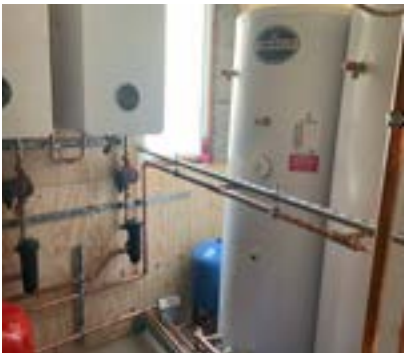
The new gas boilers and water tanks
