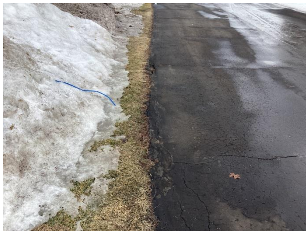
Fatigue cracks along pavement edge
