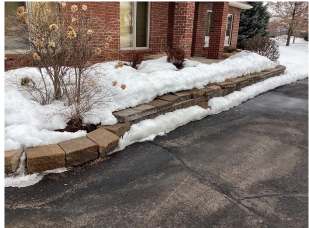
Retaining wall near Unit 117, capstone spalls and displacement evident
