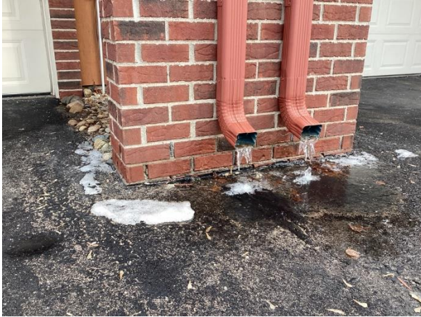
Mortar deterioration at wall base
