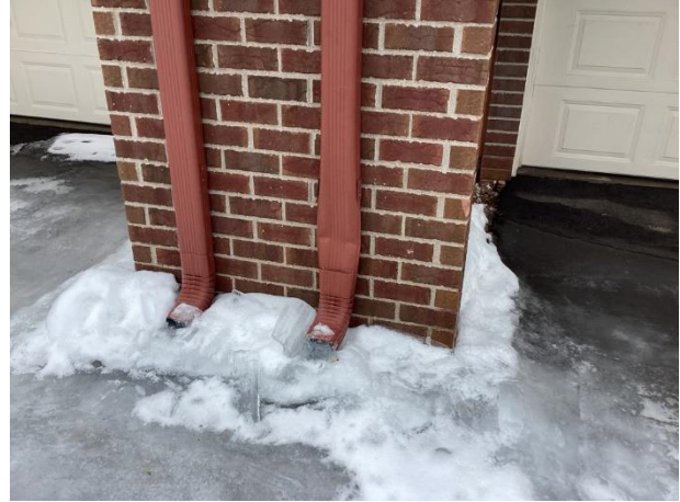
Dented downspout extension
