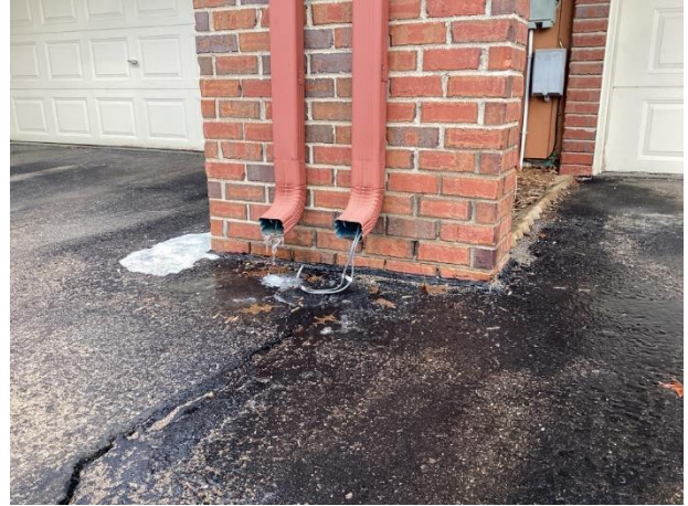
Mortar deterioration at wall base
