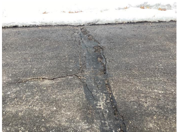
Fatigue cracks and raveling
