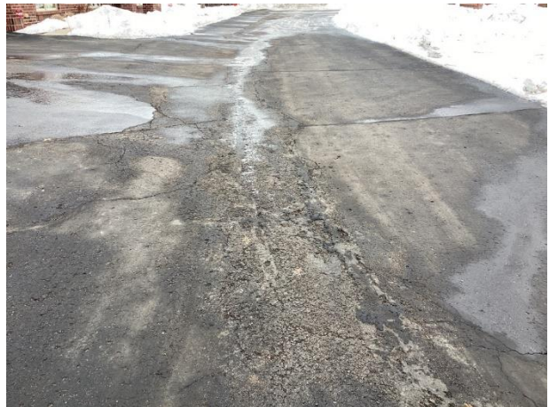
Fatigue cracks and raveling
