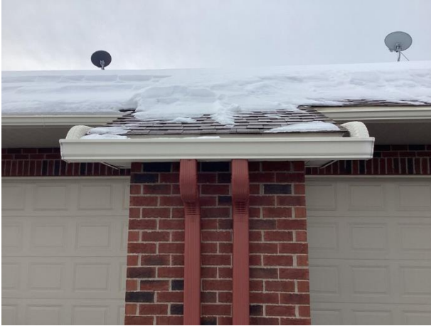
Aluminum gutter and downspouts
