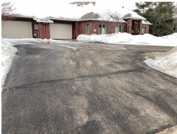
Driveway overview, fatigue cracks noted
