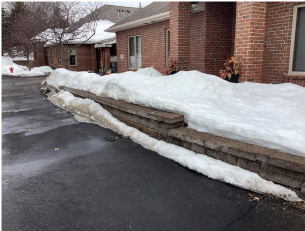
Retaining wall near Unit 133, leaning noted
