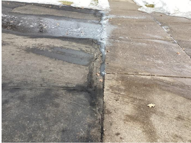
Fatigue cracks along pavement edge
