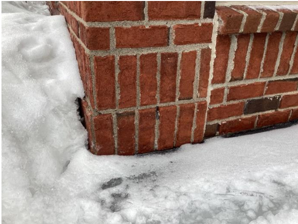
Mortar deterioration at wall base
