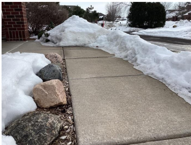
Minor sidewalk heave
