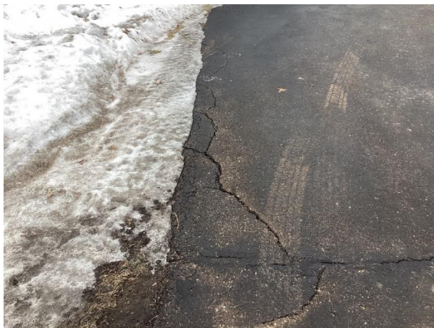
Fatigue cracks along pavement edge
