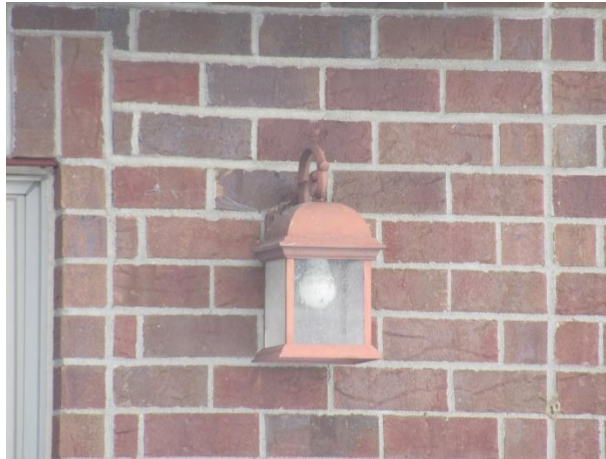
Light fixture overview
