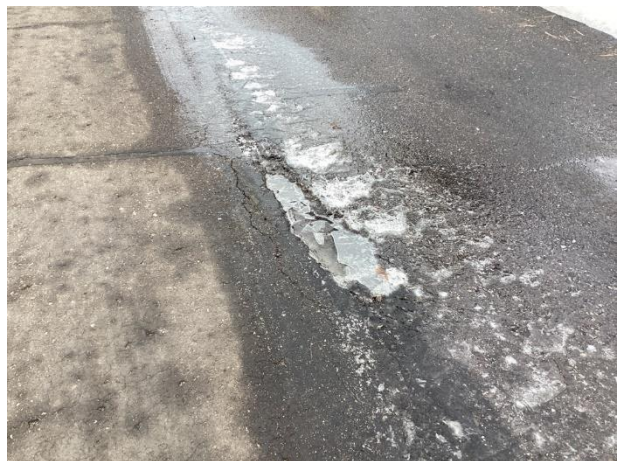
Fatigue cracks and pothole
