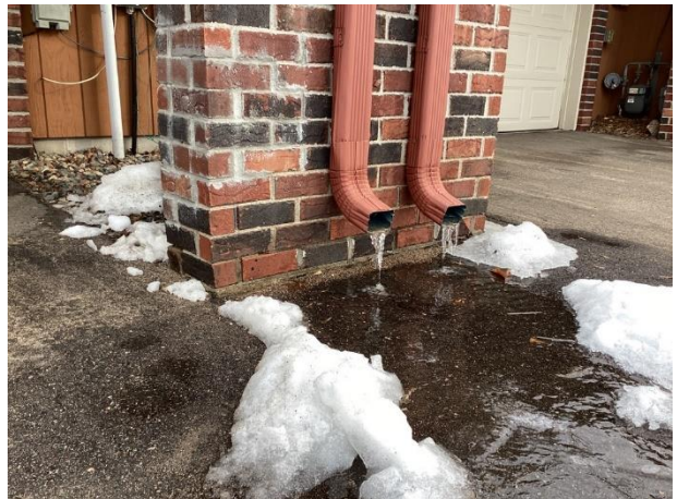
Previous mortar repairs and deterioration at wall base
