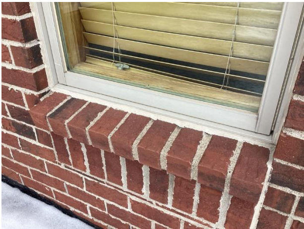
Typical window sealant. Cohesive failure at corners noted.
