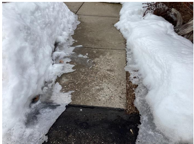
Exposed concrete aggregate
