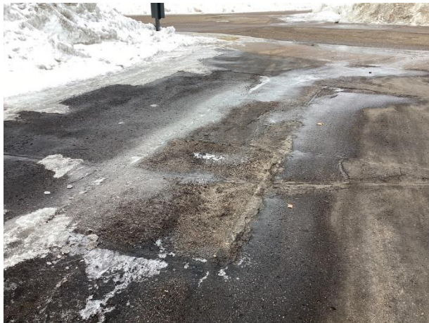
Raveling at previous pavement patch
