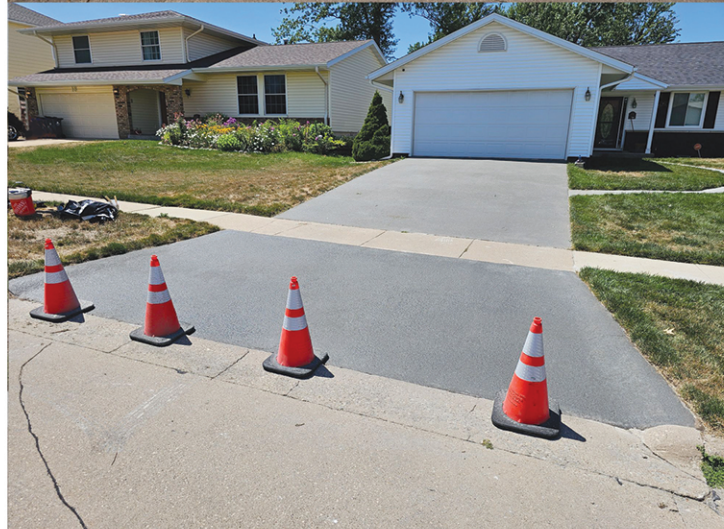
After topcoat. Final Step. You do not see the cracks. It looks like someone has poured a new slab of concrete. Not every client cares about that. Some people only want the crack to be repaired.
