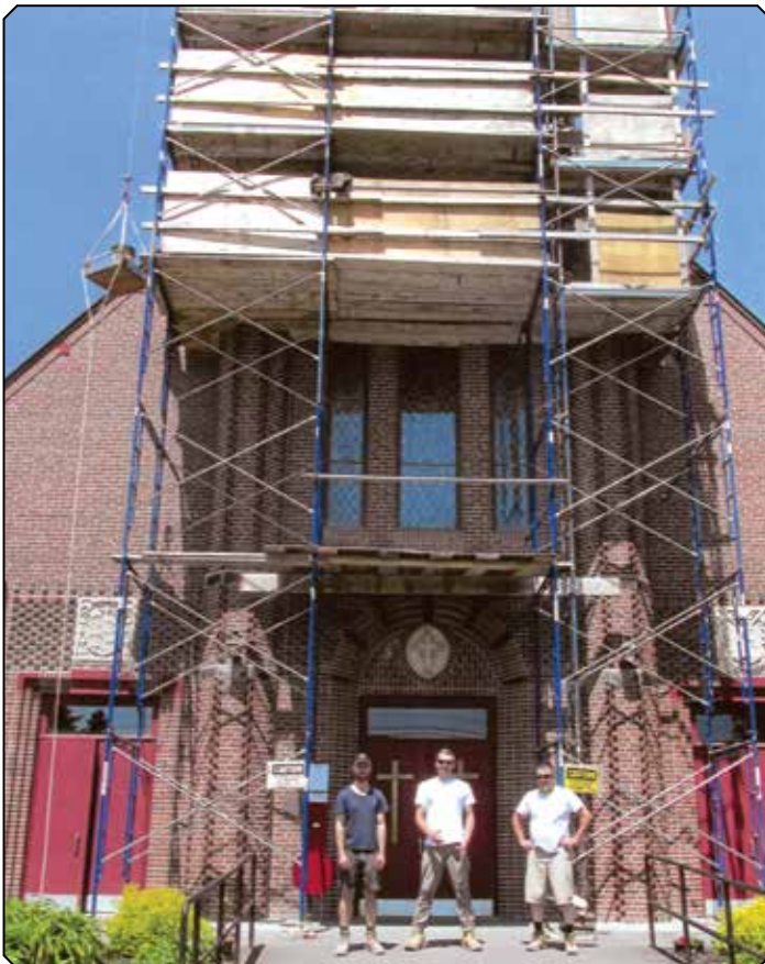
Masons from Dicon, Diocese Construction L-R: Ethan Wallace, Dakota Hood, and John Orcutt.
