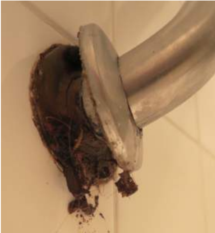
Figure 3. Corrosion behind grab bar cover plate
