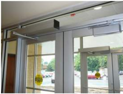
Power door operators (left doors), door closer (right door). Photo courtesy Hager Companies
