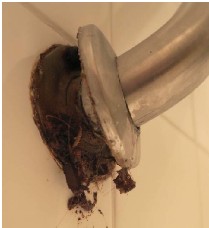
Figure 3. Corrosion behind grab bar cover plate
