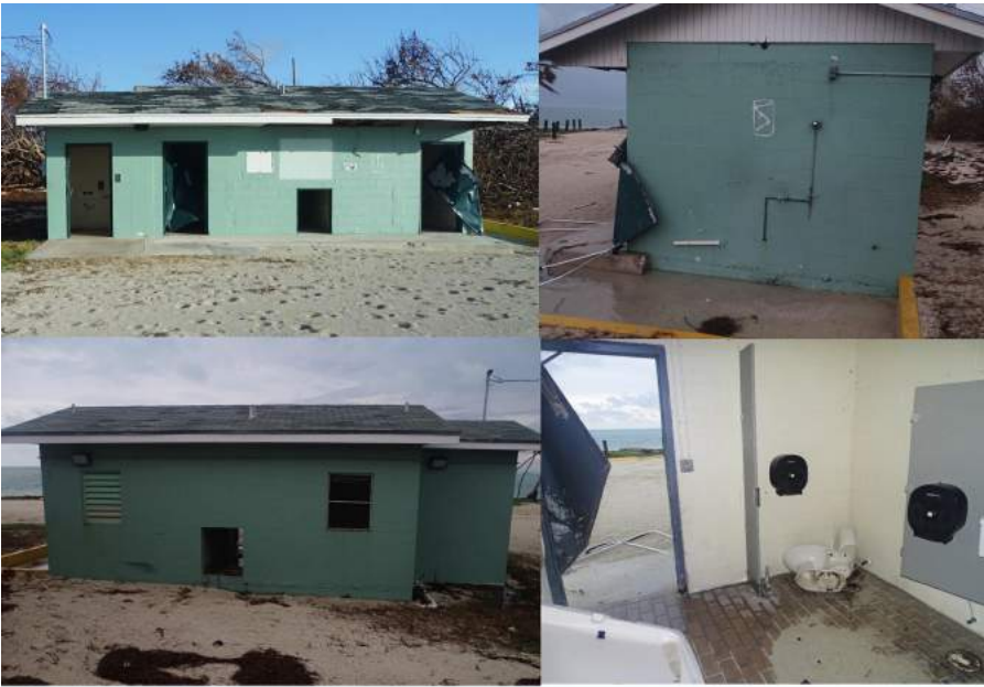
Figure 5. Florida, after Hurricane Irma, flood Zone V. No evidence of structural damage after estimated 5 ft stillwater plus waves. From upper left: facing beach, side, interior, rear.
