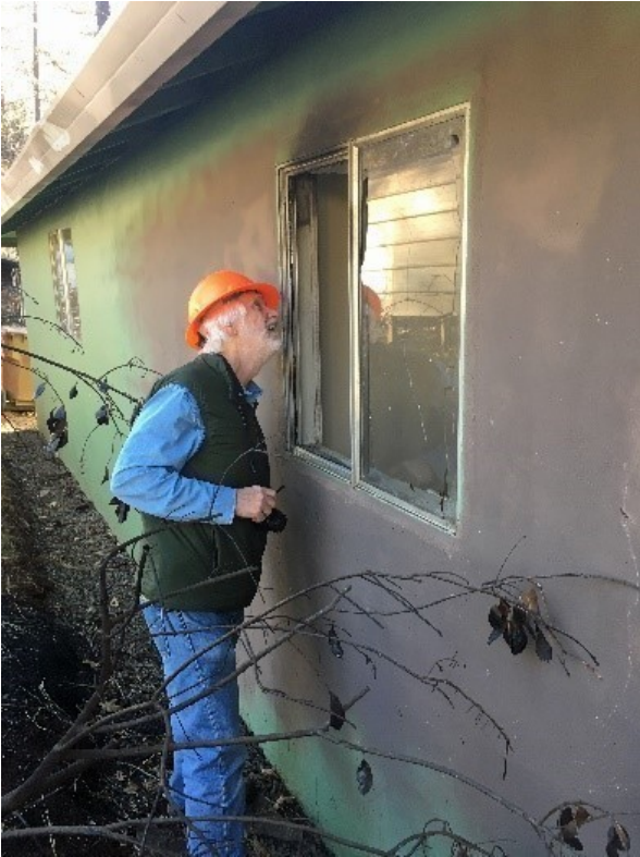
Complete failure of the glazing
