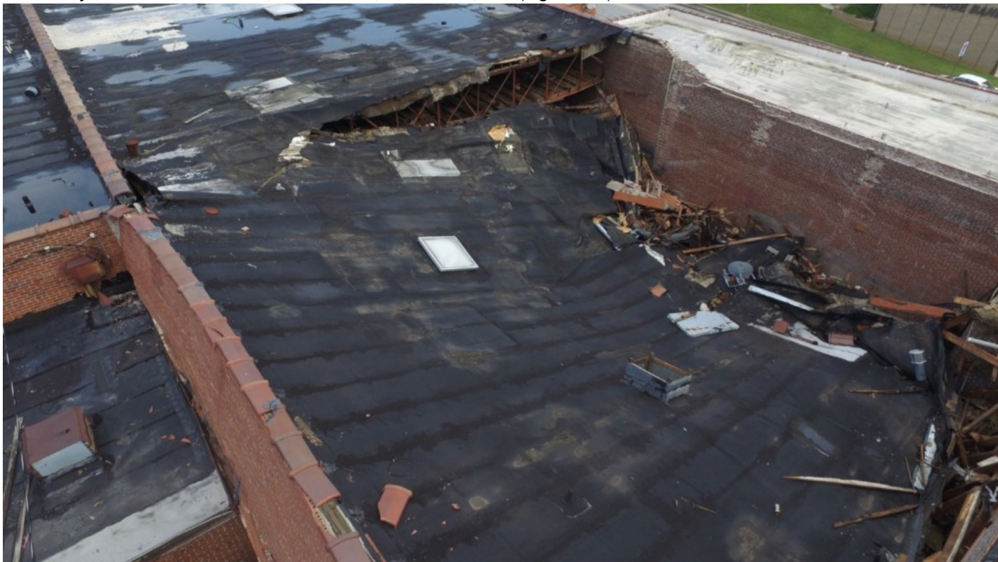
Case Study 1: Roof Failure in Walhalla, South Carolina, on October 8, 2017 (Figures 3-4)
