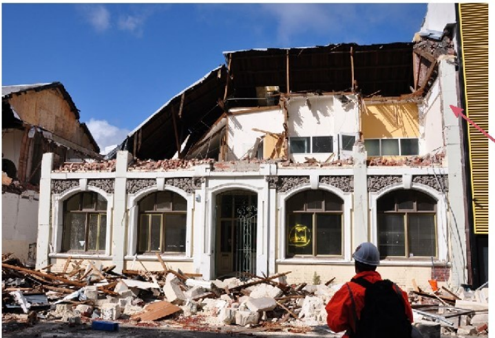
Photo of damage to masonry building in Christchurch.
