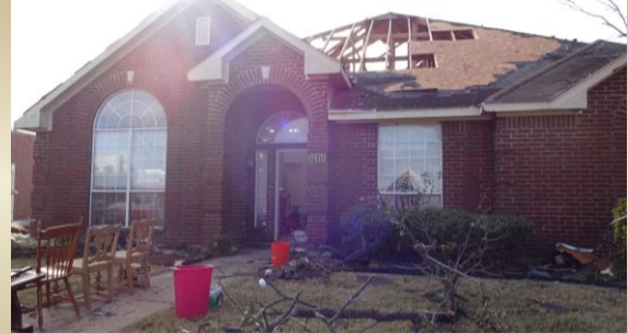
Texas Tornado – December 2015
