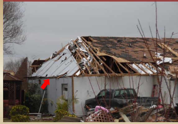
Texas Tornado – December 2015
