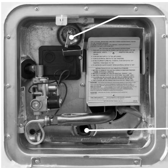
Pressure Temperature Relief Valve
