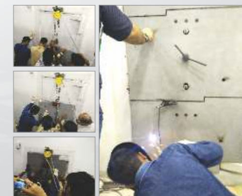
*Images from actual site installation
