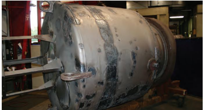
A buoy after welding. Note the band around the upper portion of the vessel approximately at the waterline – a common location of rusting/pitting.
