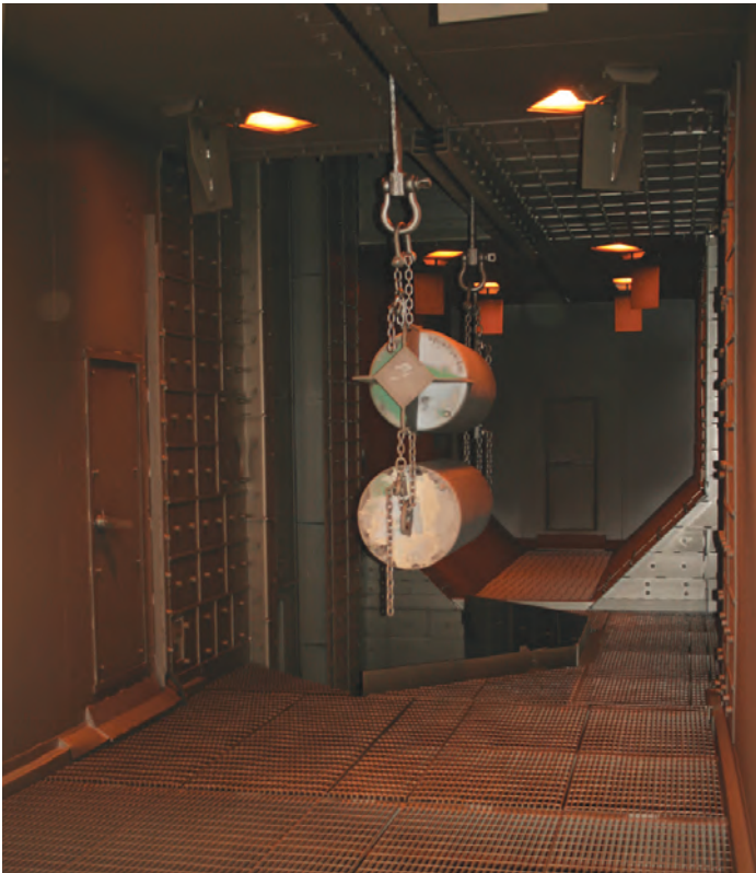
The sandblasting bay.
