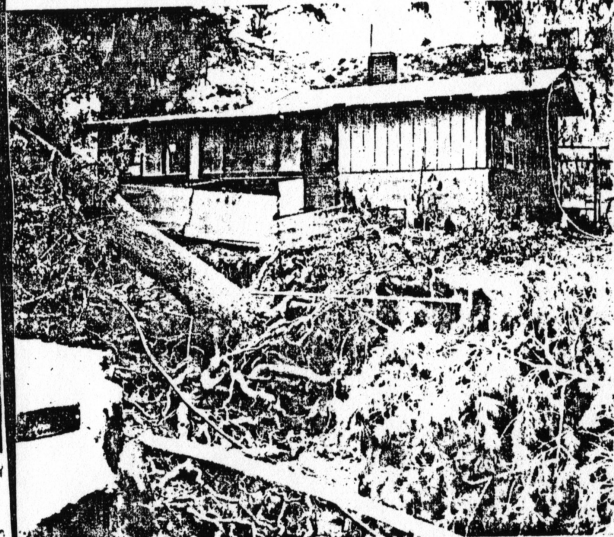
UNDERMINED — A small ranch house on the Claude Sweet property in DeLuz was undermined when a small stream became greatly enlarged and washed away part of the house's foundation. Although the structure sagged on one side the house is still being lived in.
