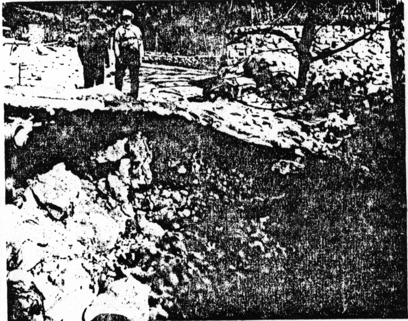
UNDERMINED CROSSING -- R. F. Matthews, left, talks with Virgil Brown concerning undermined crossing that still shows signs of damage on De Luz Creek. Some of the boulders, below, came from Vail Ranch, upstream.
