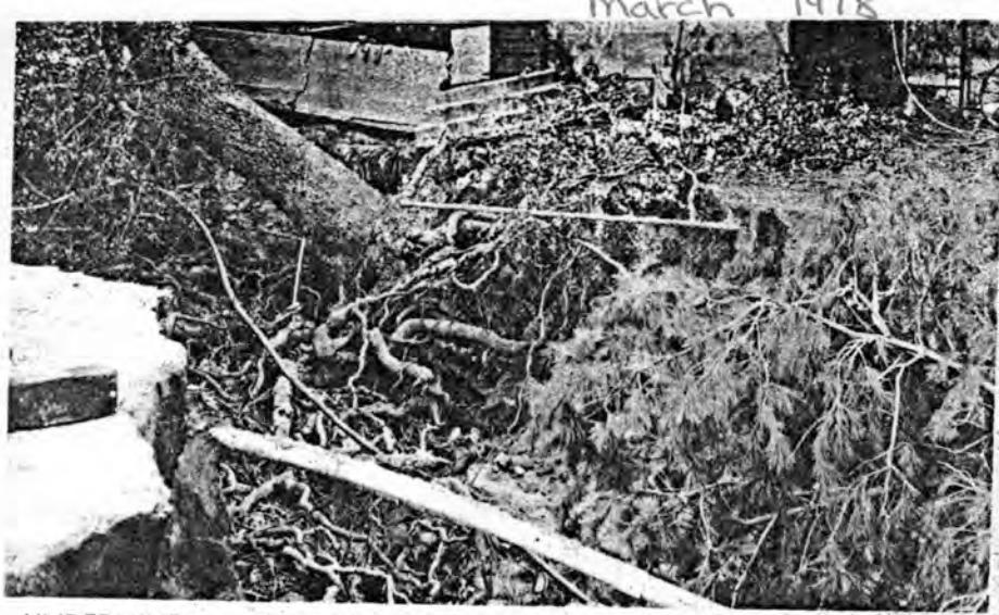
UNDERMINED — A small ranch house on the Claude Sweet property in DeLuz was undermined when a small stream became greatly enlarged and washed away part of the house's foundation. Although the structure sagged on one side the house is still being lived in.
