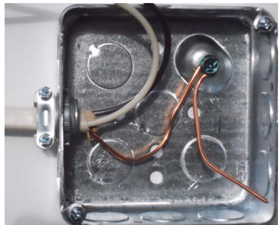
Grounding conductor attached to screw excess pig tail left to attach to receptacle etc.
