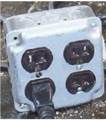
Violation of Article 405.5(C) (only one screw holding each duplex receptacle)
