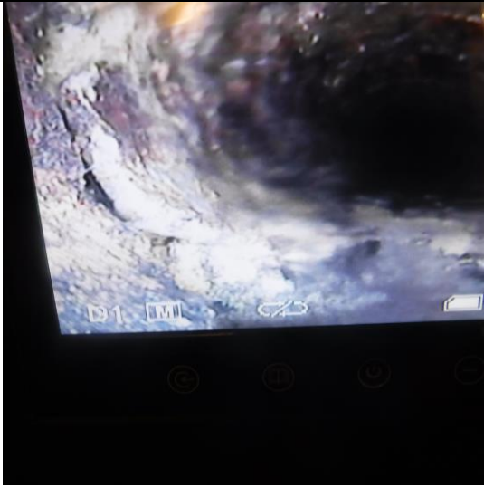
Broken cast iron line at 2 feet past front cleanout
