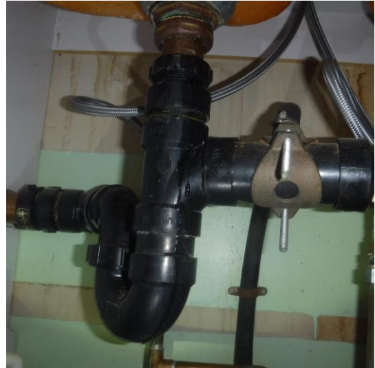
Leaking kitchen sink drain
