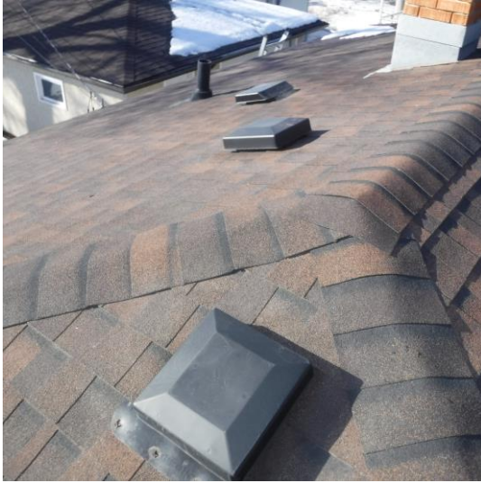
Roof top ventilation
