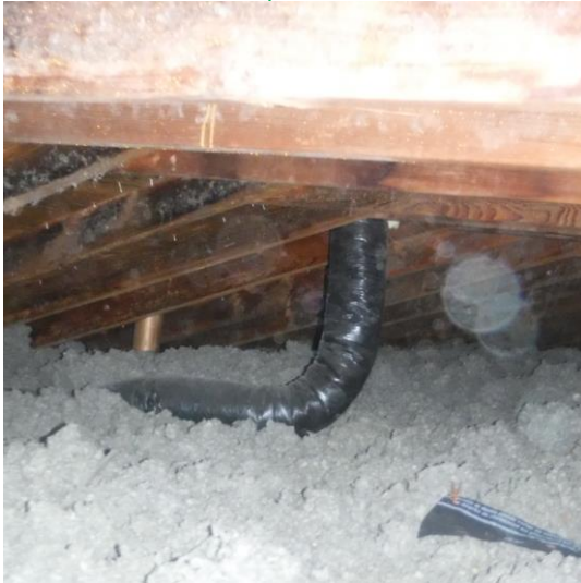
Bathroom exhaust fan termination point
