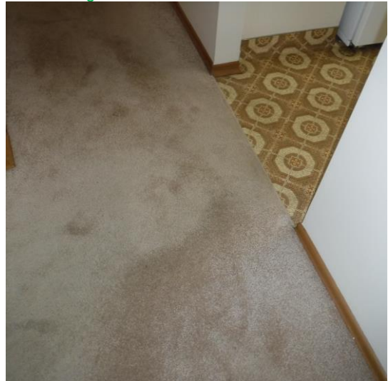
High spot sin main floor above main beam
