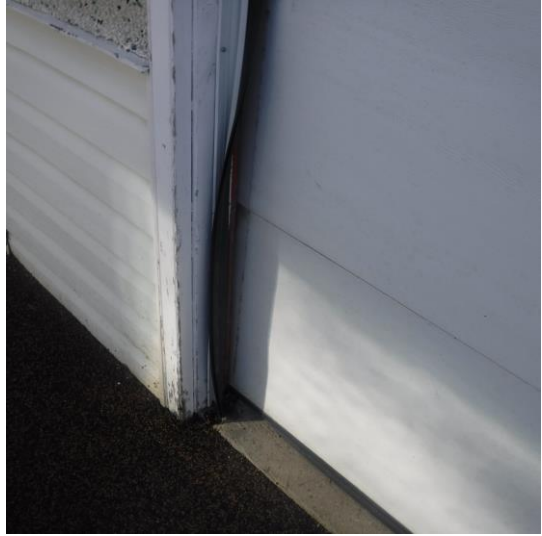
Damaged garge door seal
