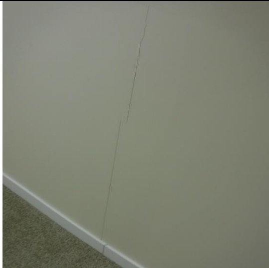
Cracking in front wall in basement drywall
