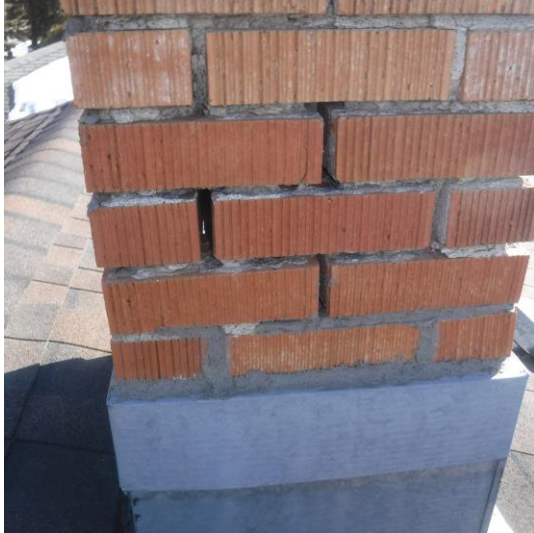
Mortar deterioration to chimney
