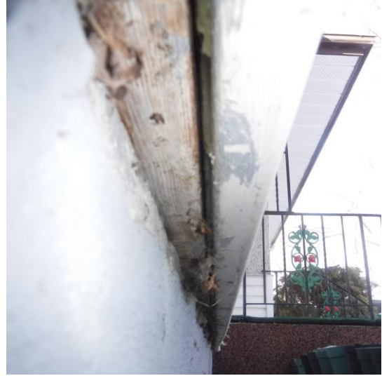
Inward movement in front foundation wall
