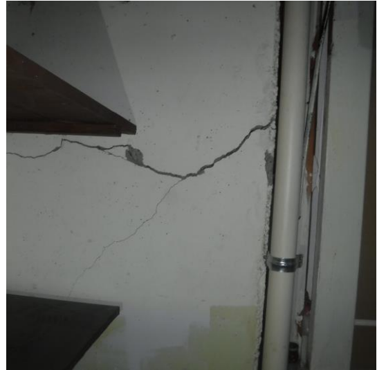
Cracking in front foundation wall
