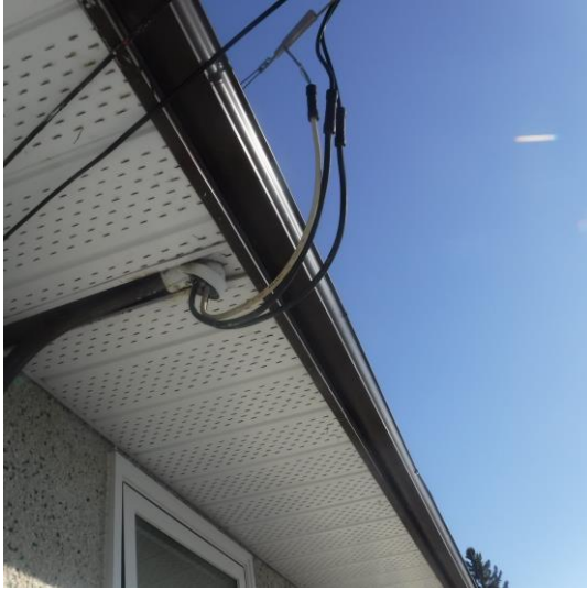
Service entrance-mast head
