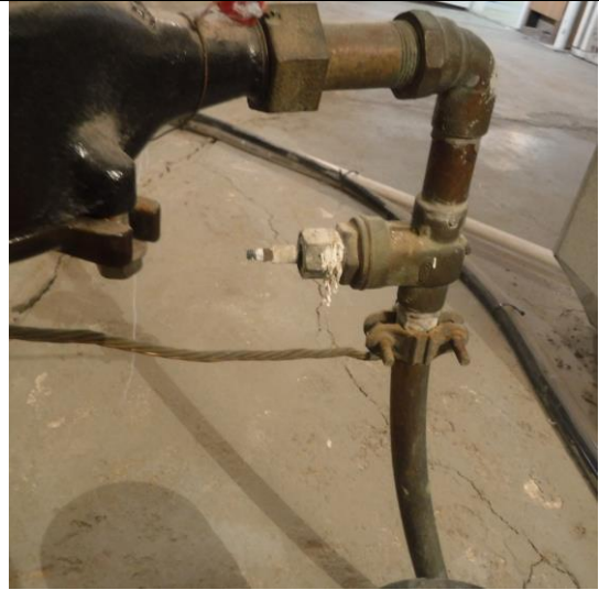
Missing shut off handle on main water line
