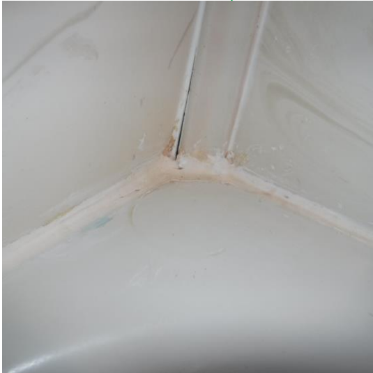
Unsealed tub surround
