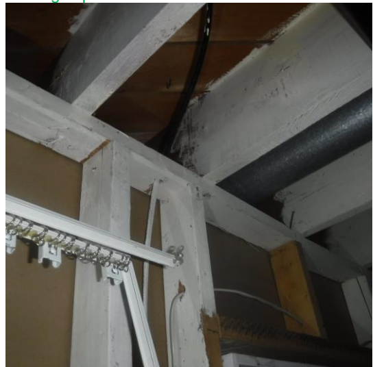
Un-floated basement walls
