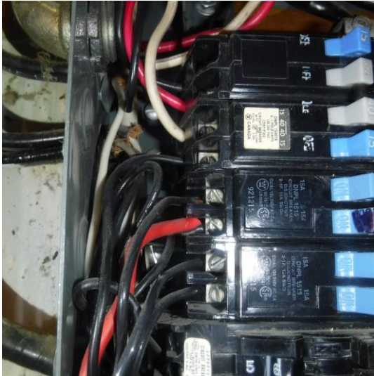
Double tapped breaker in panel
