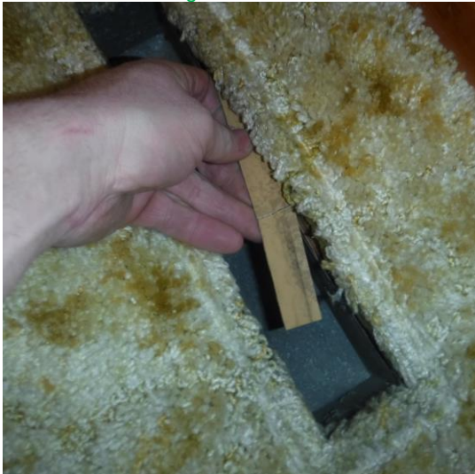
Possible asbestos flooring
