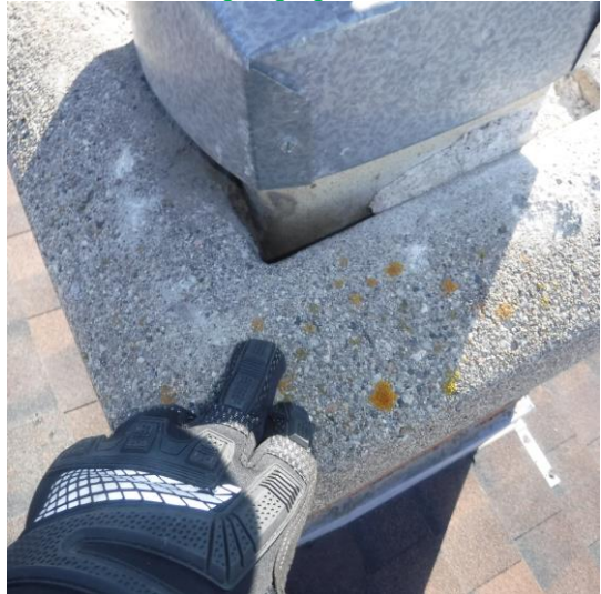
Unsealed chimney cap
