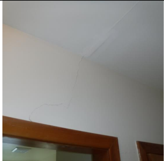
Cracking in main floor walls/ceilings
