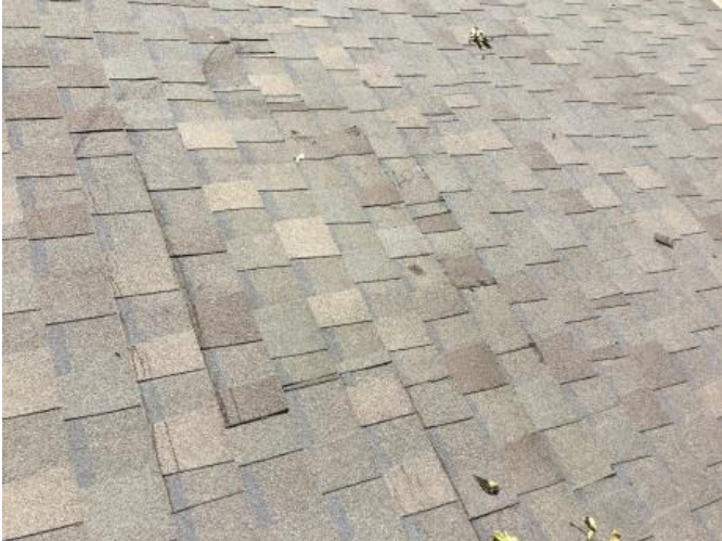
Minor tree damage to shingles
