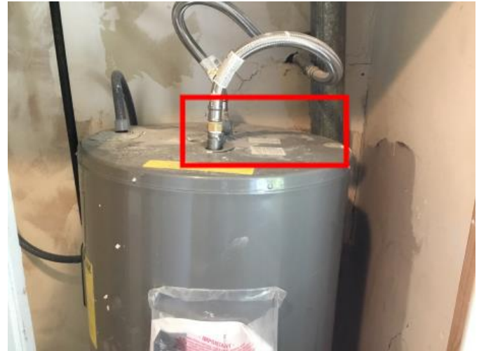
No TPR overflow pipe
