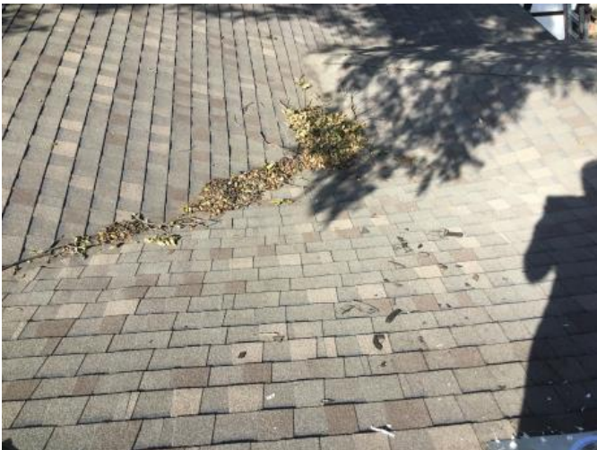
Debris in valley
