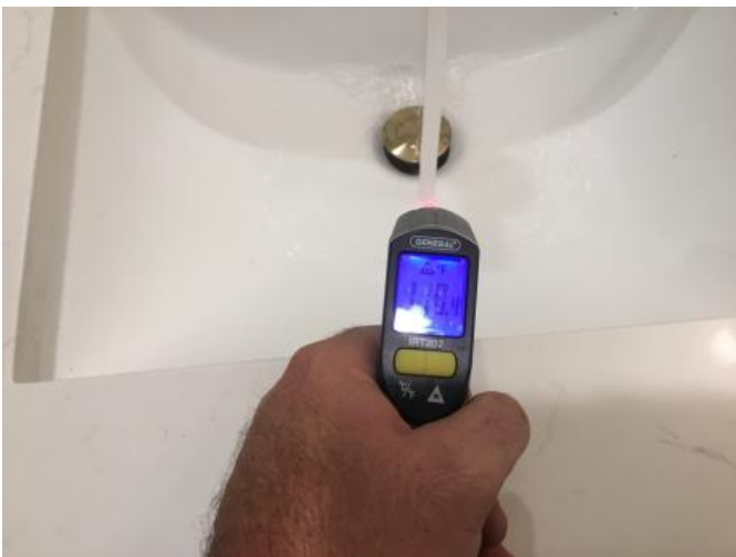
Hot water measured at 118 degrees.
