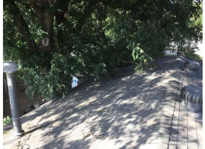
Trees contacting roof
