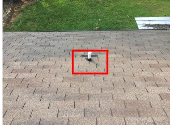
Vent sealing deteriorating
