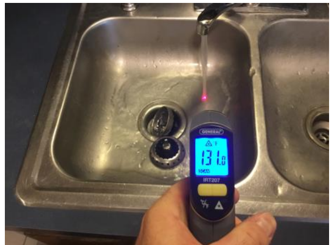
Hot water measured at 131 degrees
