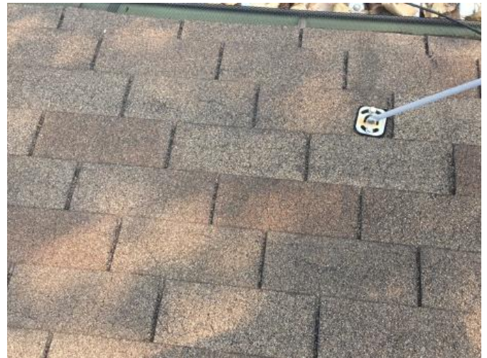
Cracking and Loss of Granules
