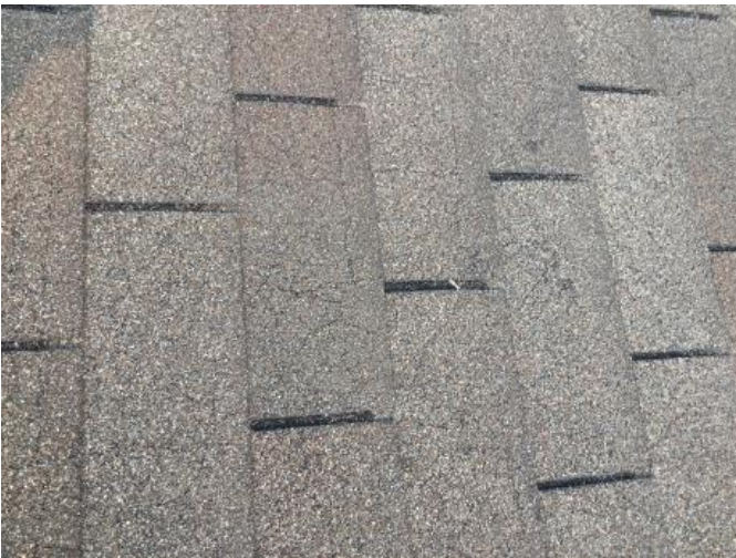
Cracking and Loss of Granules
