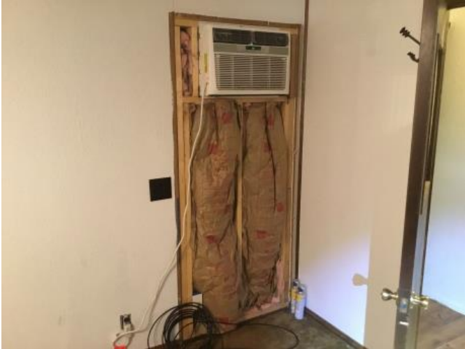
No drywall installed
