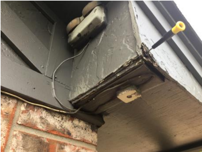
Moisture damage on fascia
