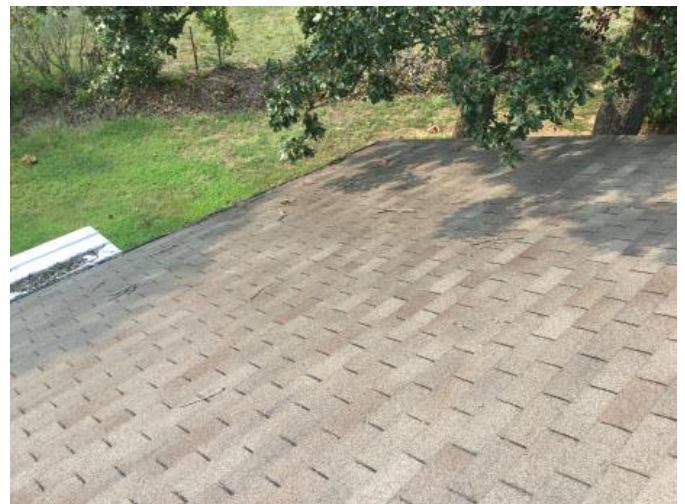
Debris on roof
