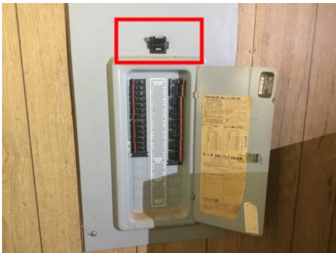
Main disconnect in the house
