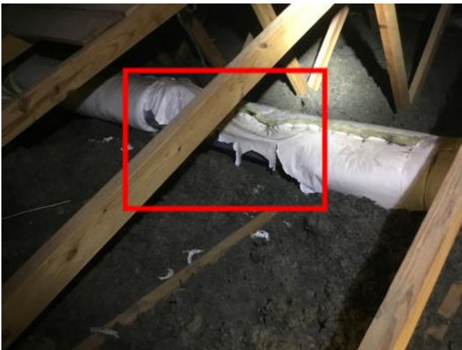
Duct insulation damaged
