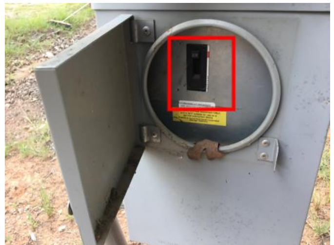
Main disconnect at the pole
