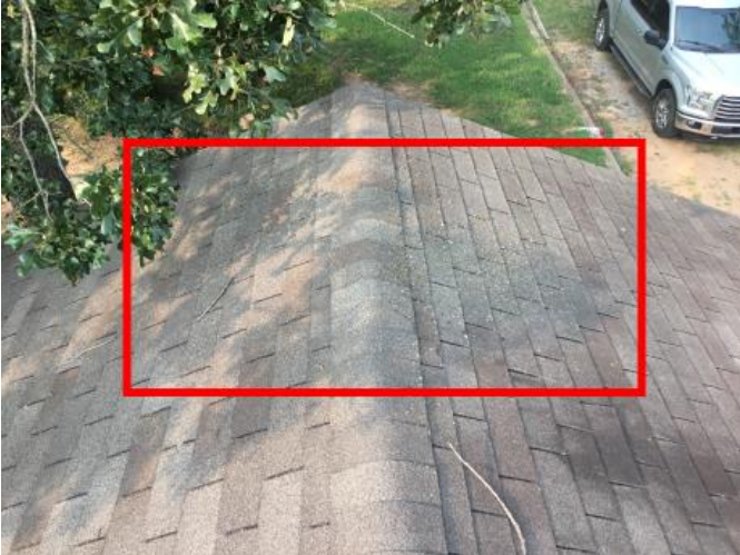
Moss on roof under tree
