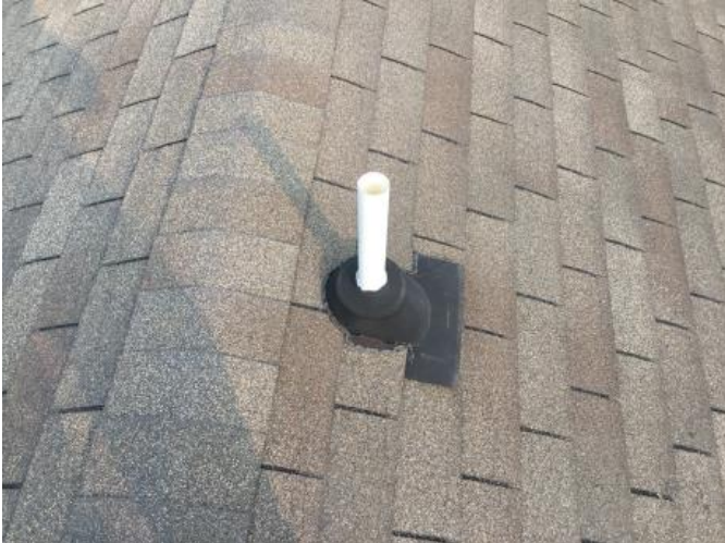
Vent sealing deteriorating
