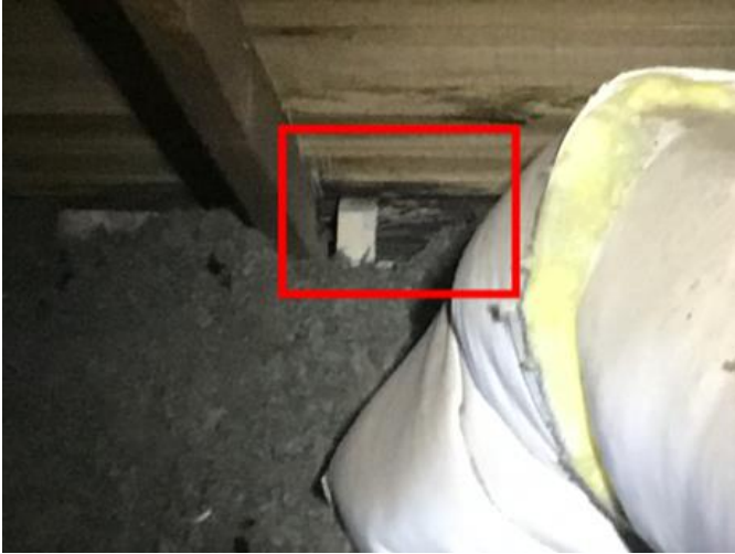
Water stains by chimney
