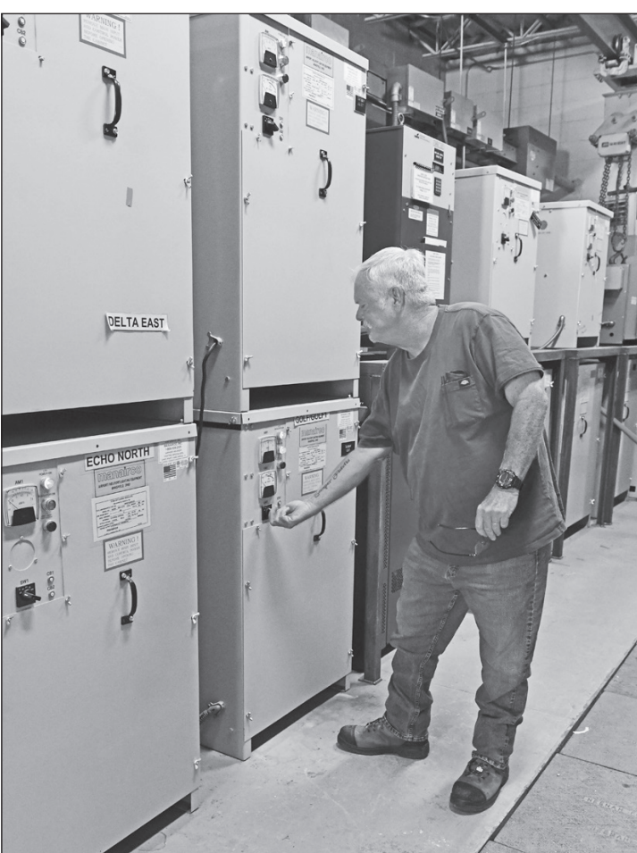
Robby Lane, 78th CES Facilities Flight high voltage electrician, checks the switch of an airfield lighting regulator at Robins Air Force Base, Georgia, June 28, 2023. Multiple lighting regulators are used to control the various airfield lights across the flight line, taxiways and the runway. (U.S. Air Force photo by Joseph Mather)
