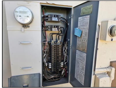
Deadfront Removed and Service Disconnect
