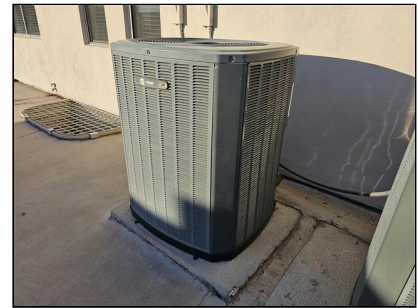
Heat Pump #2 Trane 5 Ton
