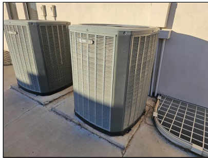
Heat Pump #1 Trane 5 Ton
