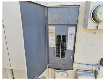
Electrical Service Panel
