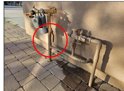
Main Water Shut Off Valve
