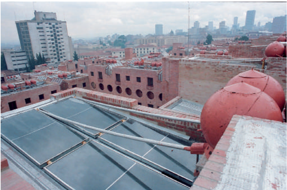
GAVIOTAS solar water heaters in Nueva Santa Fé condominium
