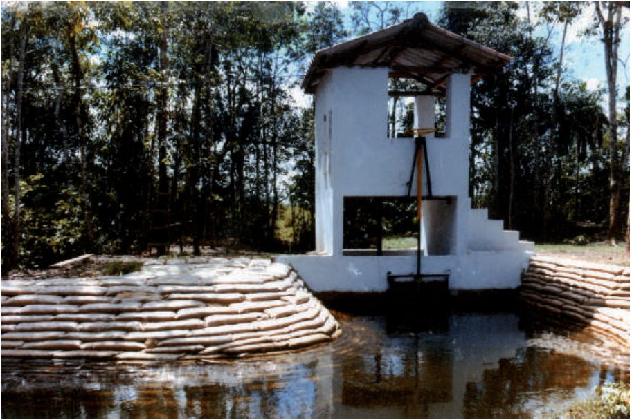
Dam and powerhouse of GAVIOTAS hydraulic electric turbine to generate electricity with low waterfall
