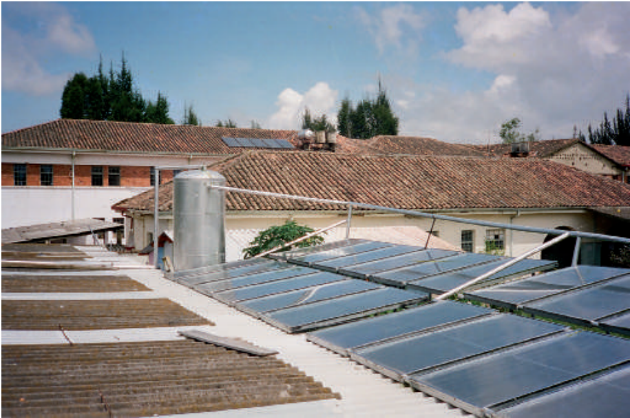
GAVIOTAS solar heaters installation in an elderly home
