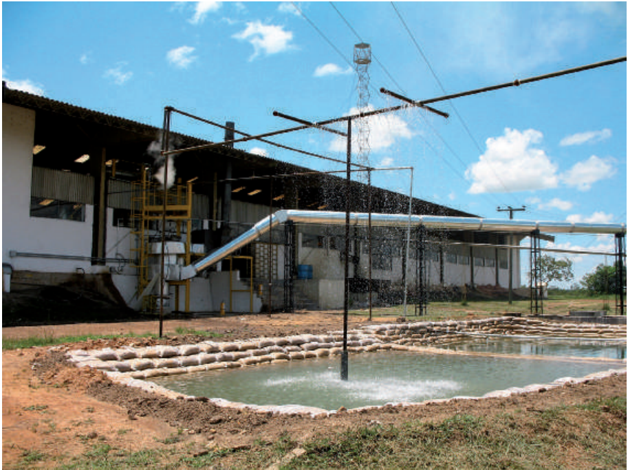
Aspect of the generation of electricity from the GAVIOTAS rosin plant. In these ponds cachamas, native fish Orinoquia are being cultivated
