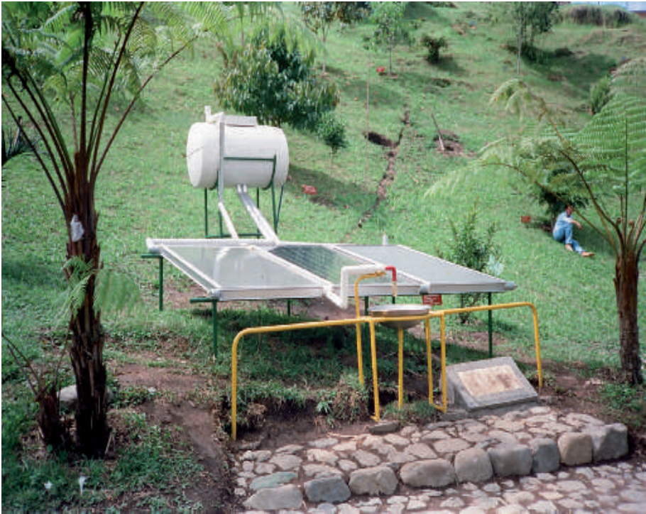
Solar interactive module for water heating made by GAVIOTAS
