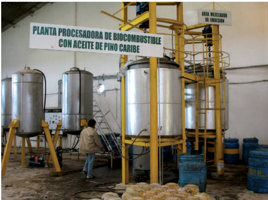
Overview of pine oil biofuel processing plant
