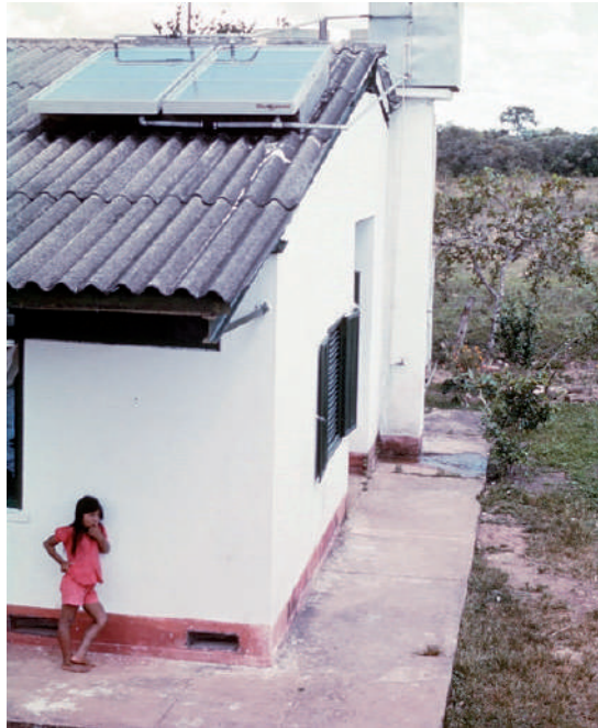
First GAVIOTAS solar water heater in Vichada
