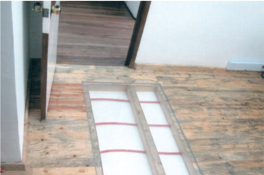
Solar space heating by radiant floor in GAVIOTAS office in Bogota
