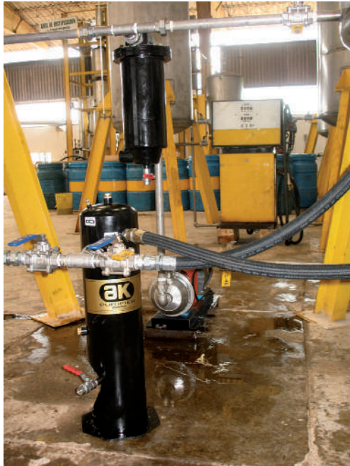
Detail of biofuel processing plant pine oil
