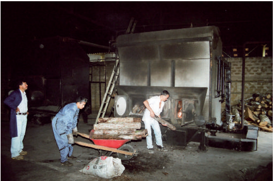
Boilers fueled by wood logs from pruning and thinning the forest, GAVIOTAS
