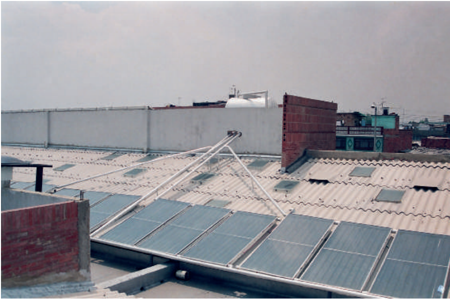
GAVIOTAS solar heaters installation in a health care center from social security, Bogota
