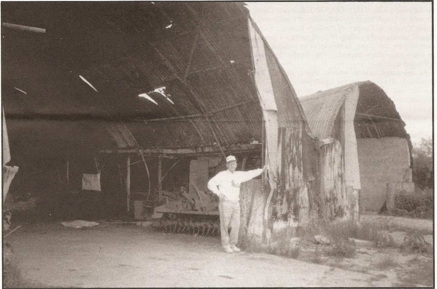
It is said that a picture is worth a thousand words, how true that is in this instance. The picture of a pair of badly deteriorated huts 56 years after erection still shows evidence of former glory as wartime depot warehouses. Initially these buildings were rumored for chemical warfare storage. These pictures are proof too of civilian acquired construction skills of the hard working 107 th men. The picture, contributed by the posed Paul J. Van Abel [E/107 NG, Calumet], was taken during "Van's" '98 revisit during which he exchanged informative particulars with the present landowner.
