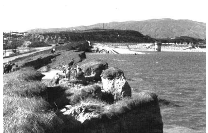
Figure 41 - Lower San Fernando Dam that was badly damaged by the 1971 San Fernando Earthquake.
