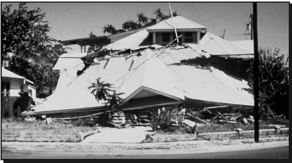
Additional damage from aftershocks
