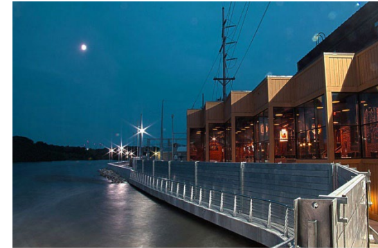
PERIMETER FLOOD BARRIER
