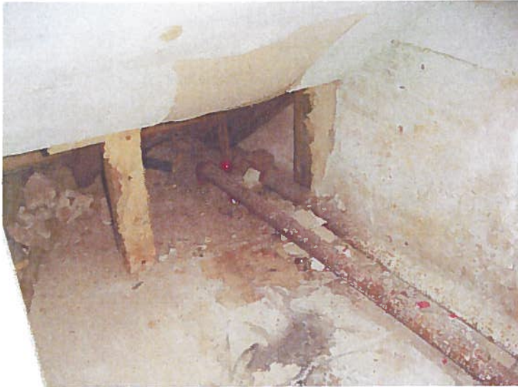
Photo 16 – Under a stairwell inside the Chestertown Armory building located at 509 Cross Street in Chestertown, Maryland.
