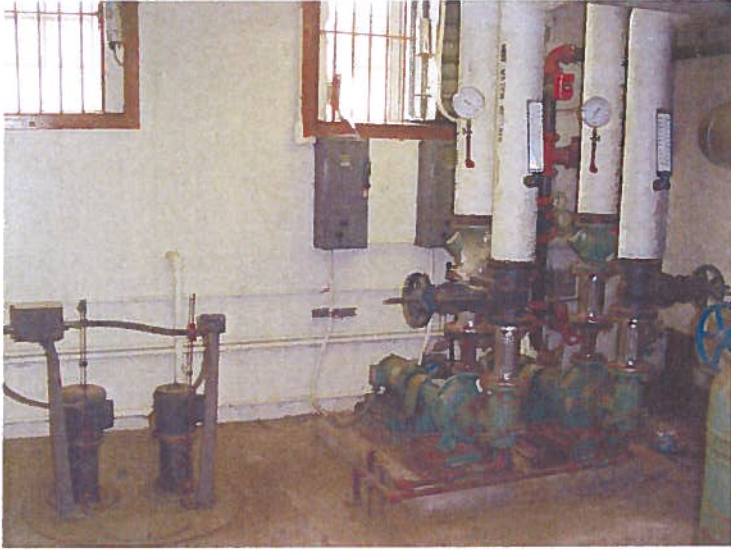
Photo 21 – View of the circulation pumps inside the boiler room of the Chestertown Armory building located at 509 Cross Street in Chestertown, Maryland.
