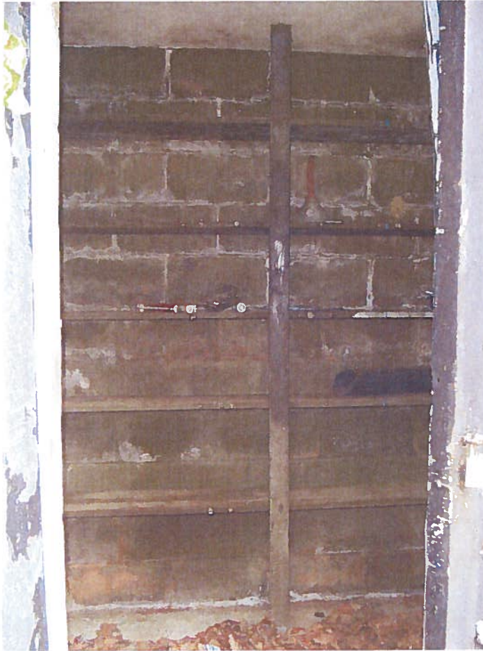
Photo 25 – Inside view of the small block building identified as “POC” along the south edge of the Chestertown Armory property located at 509 Cross Street in Chestertown, Maryland.
