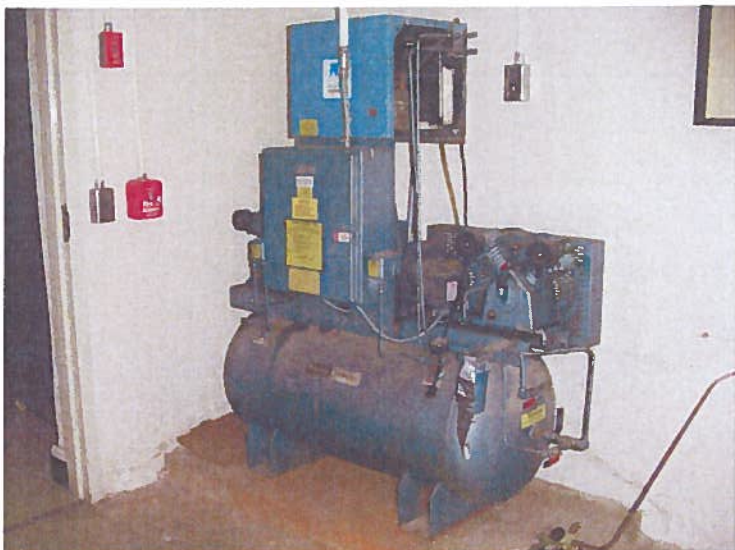
Photo 18 – View of the air compressor in the boiler room of the Chestertown Armory building located at 509 Cross Street in Chestertown, Maryland.
