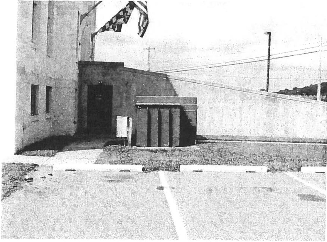
Armory power transformer located on front east side of the building.
