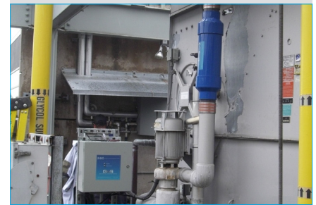
General Water Systems' Sustainable Water Treatment
