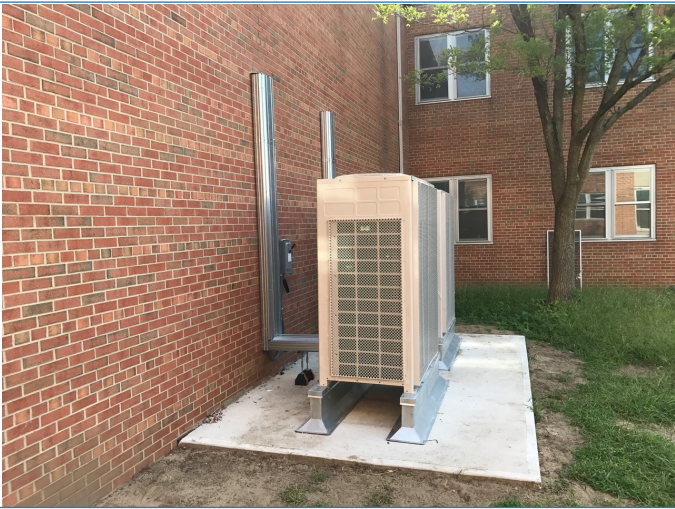
VRF System installed by the wall with Slimduct RD running vertically
