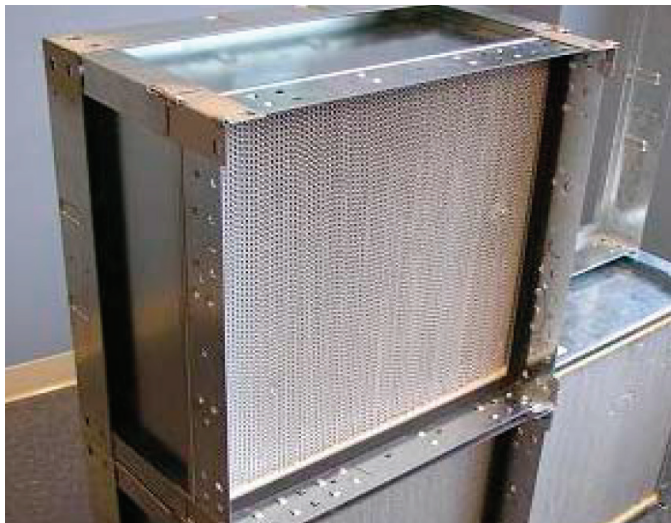
Figure 46: Properly Installed HEPA Filter
