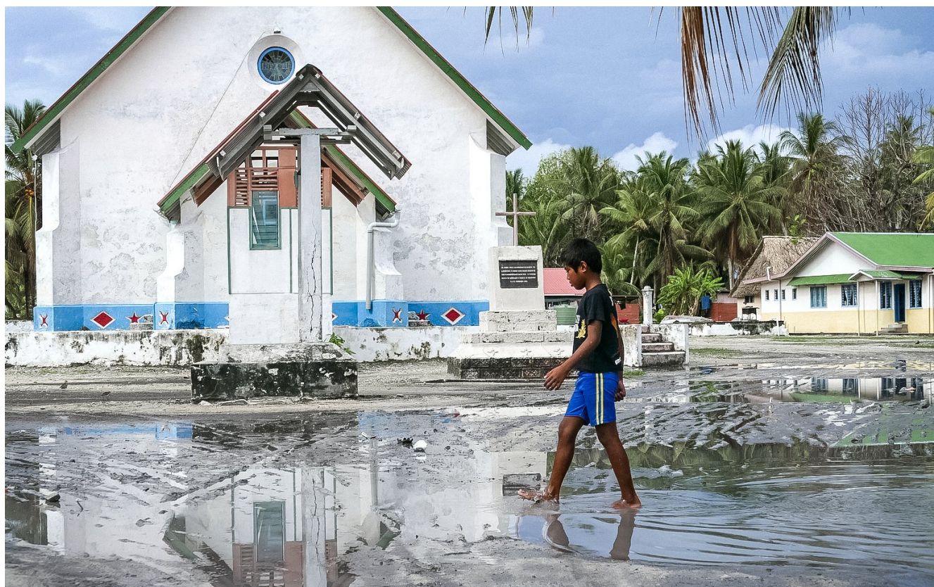
A child in Tuvalu walks through damage from Cyclone Pam. Photo by Silke von Brockhausen / UNDP (CC BY-NC-ND 2.0)
