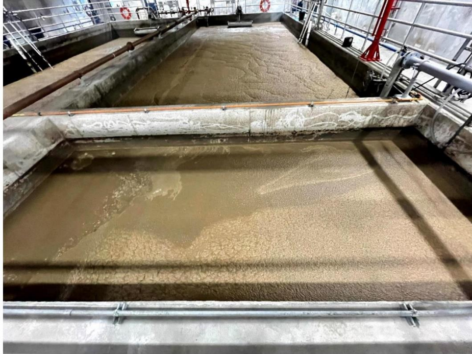
Figure 2: One of the pre-react zones showing floating FOG and some foam accumulating.
