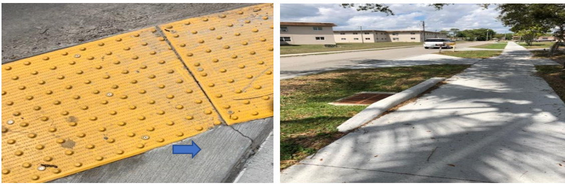
03.17.22 crack under ADA mat NE corner of Eustis/S 5 th and S 5 th St requires a handrail on stem wall
