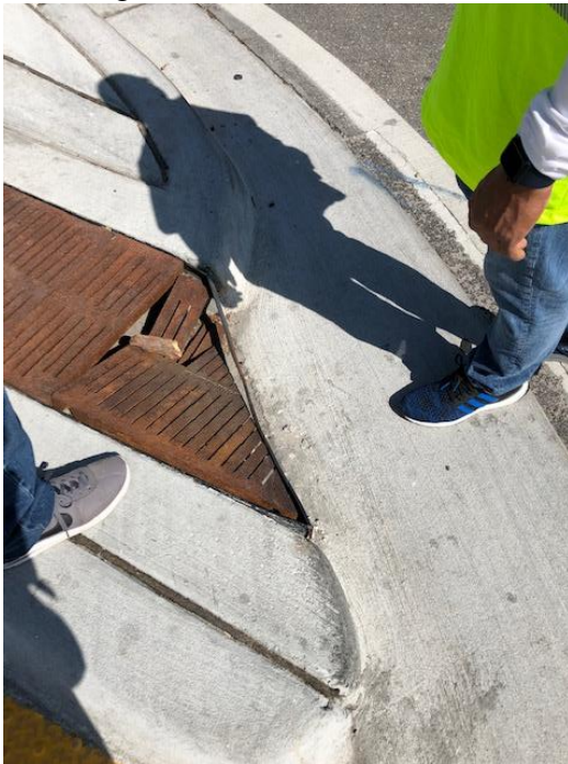
Broken grate S 2 nd St - 4.5.21
