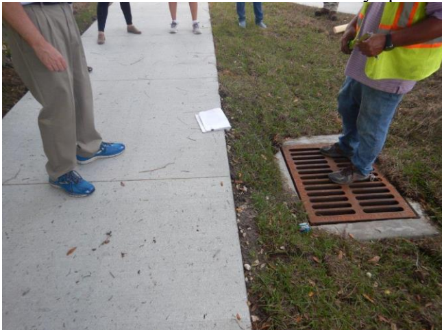
BEFORE: Condition of sidewalk 2' safety space at Final Walk Through
