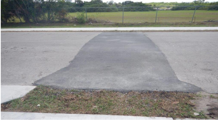
BEFORE: Condition of open cut on Carver at Final Walk Through
