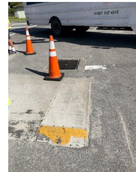
12.3.21 Replacement needed of ADA Pads
