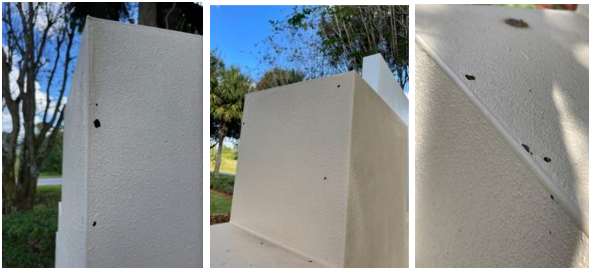
Stucco Failure at Triangle Monument 11.16.21
