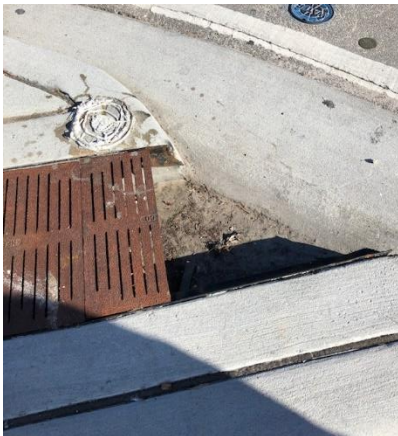
SW corner of 4st S & W Main damaged grate
