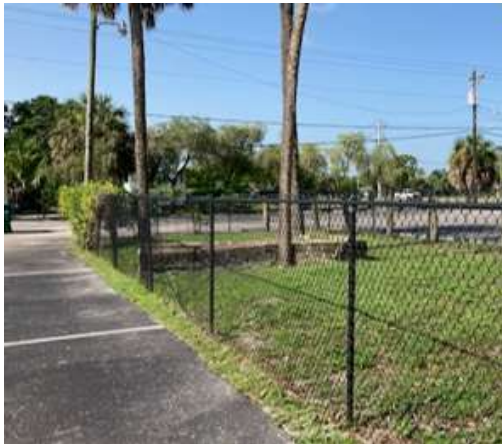
07.10.23 Fence line sagging
